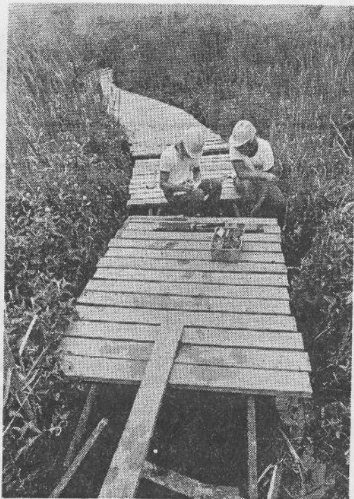
Alan Lassman, left, and John Lein, work on a boardwalk that will carry visitors into a swampy section of Huntley Meadows Park in Fairfax County. At right,
