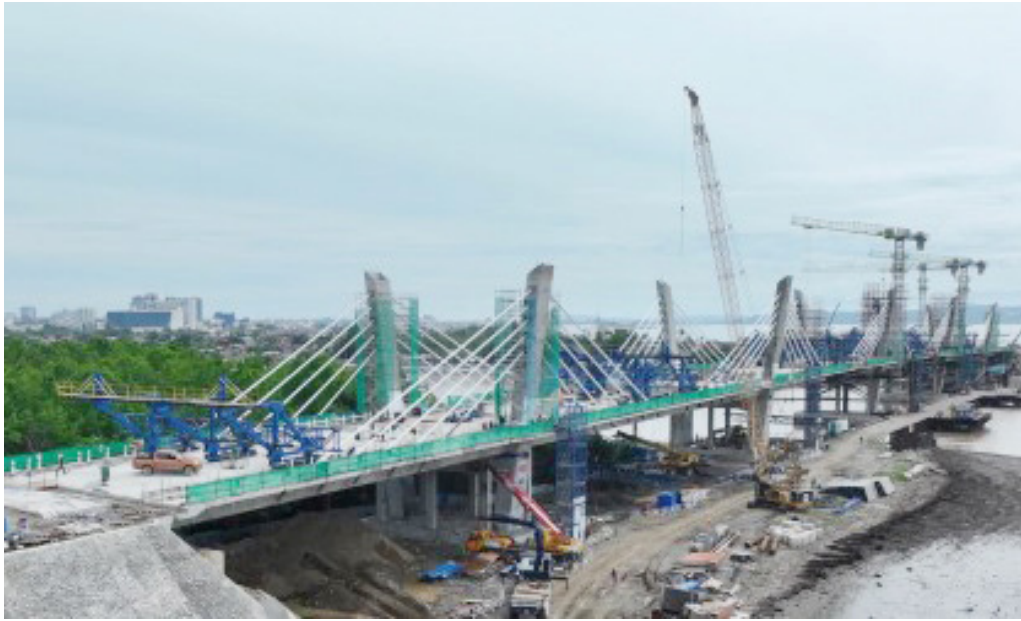
KEY PROJECT. Construction is in full swing at the Bucana Bridge Project in Davao City in this photo released by the Department of Public Works and Highways (DPWH) on Friday (June 27, 2025). The construction of the PHP3.126-billion project is expected to reach 95-percent completion by July. (Photo courtesy of DPWH)
