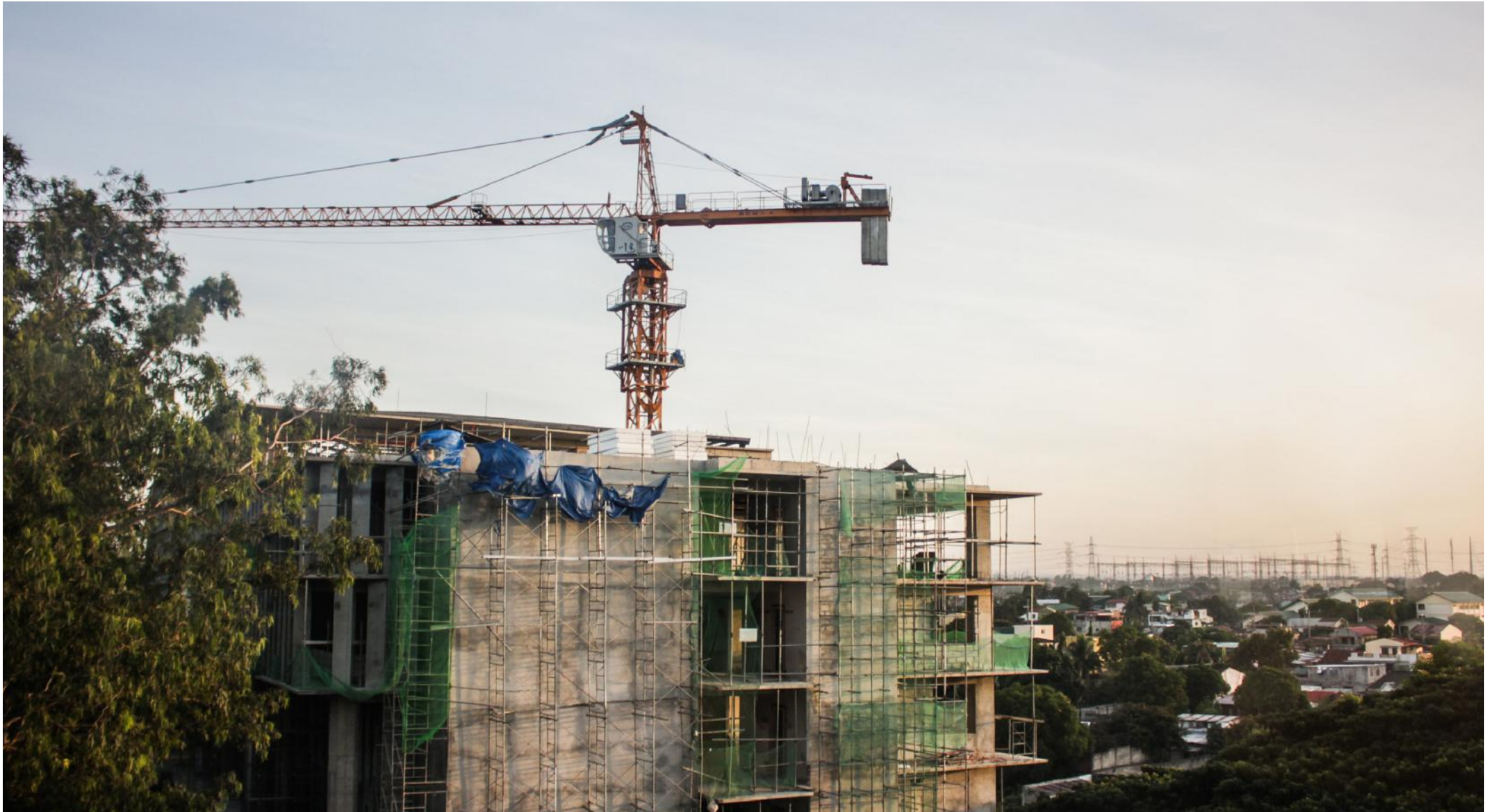
TOPPING OFF. Due to inclement weather and design adjustments, completion of the new CEAT building prolongs until next year after its topping off ceremony on September 12. | Photo by Jean Quinto
