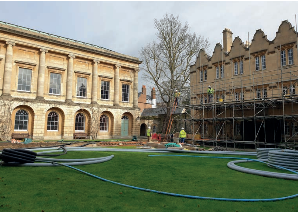
Extensive restoration works to Staircase 8 during Hilary Term were interrupted by lockdown
