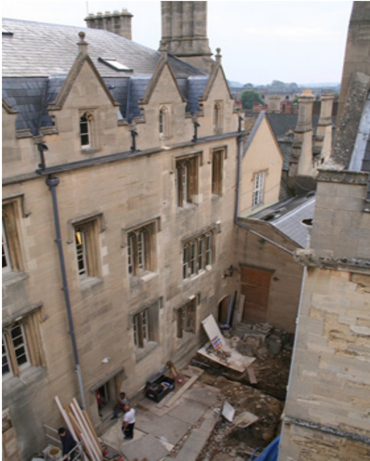
Aerial View of Staircase 8, from North Quad, September 2005 Note the toilet block has been demolished
