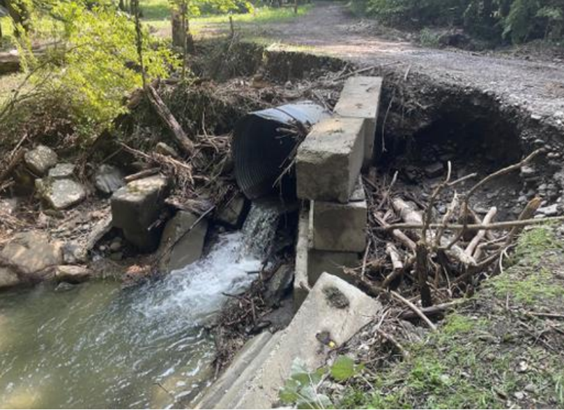
Before: An undersized culvert caused floodwaters from a 5-inch rainfall event to wash away sections of Reservoir Road, the only access to the Village of Naples Water Treatment Plant
