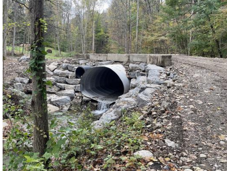
After: A much larger culvert and 200 feet of stabilized streambank now help manage peak storm flows and reduce the risk of future flooding
