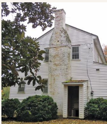
Griffin-White House, Pittsboro vicinity, Chatham County. 1830s. Early Federal/Greek Revival house. Easement Donor: Blandford Frothingham, LLC, Pittsboro.
