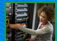
NETWORKING AND LOW-VOLTAGE INSTALLATION & SERVICE
