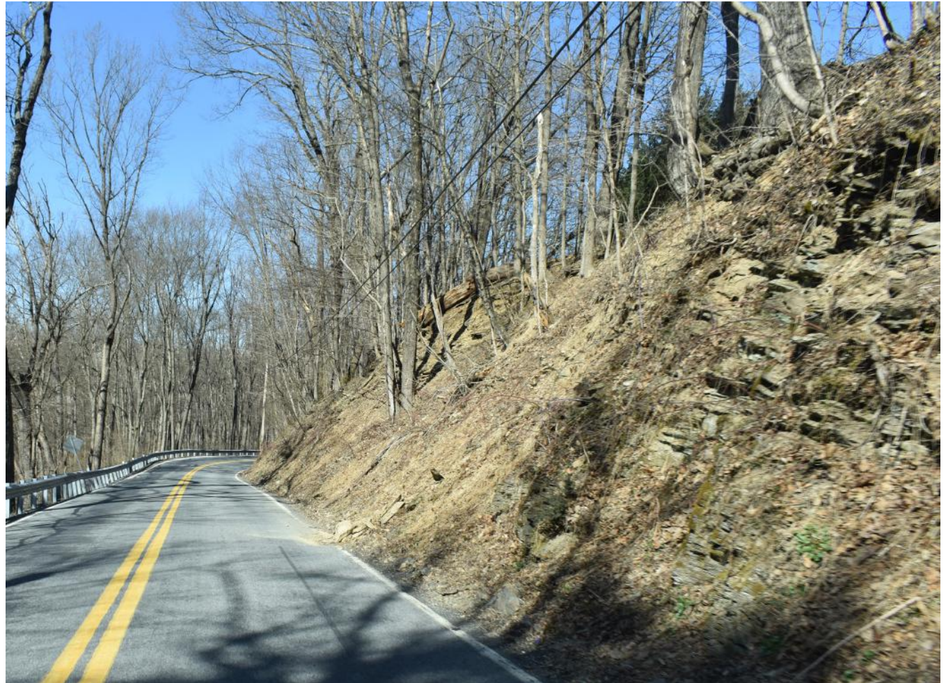
Steep slopes along roadway | Source: South Whitehall Township
