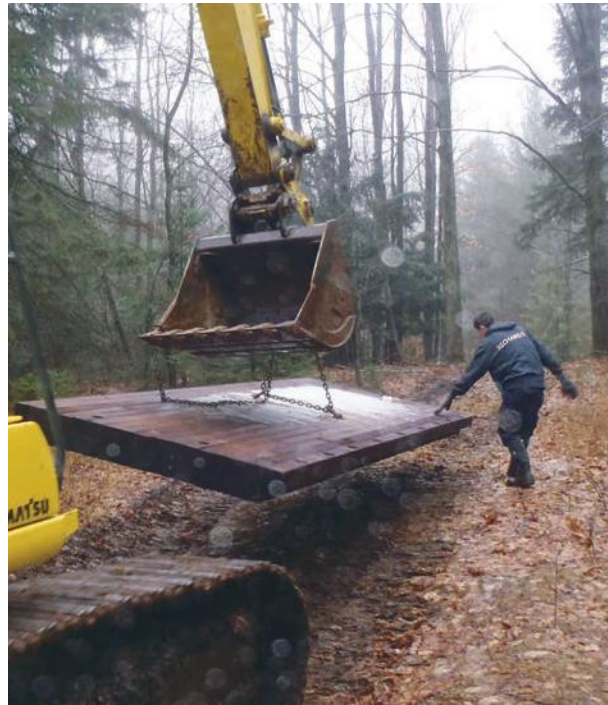
The deck for the timber bridge is delivered replacing a failed culvert on Bancroft Creek.
