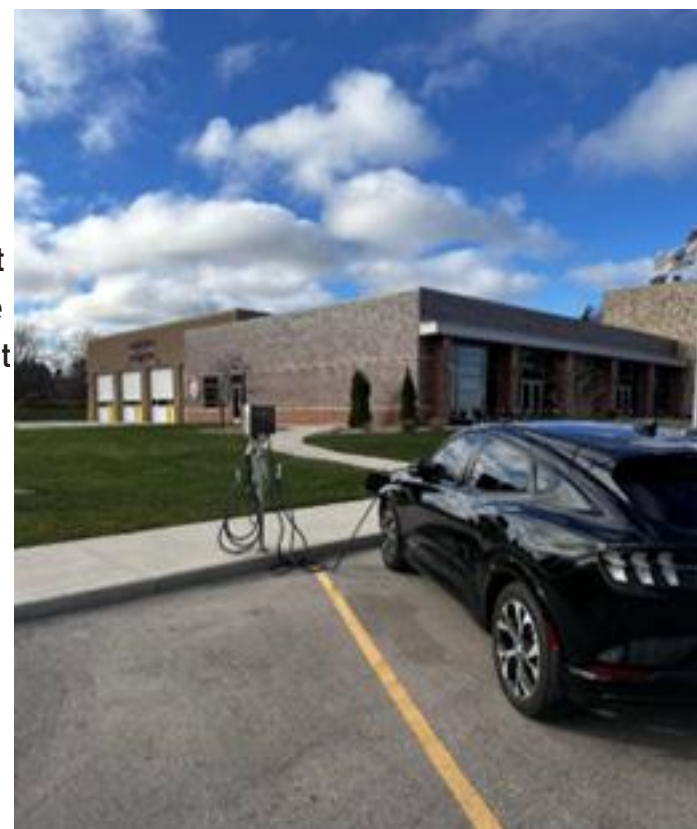
Figure 3.25: Town of Ledgeview Town Hall EV Charging Station
