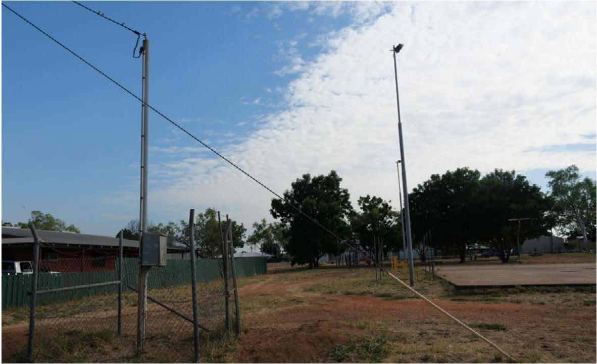
Figure 65: Power box located near the courts
