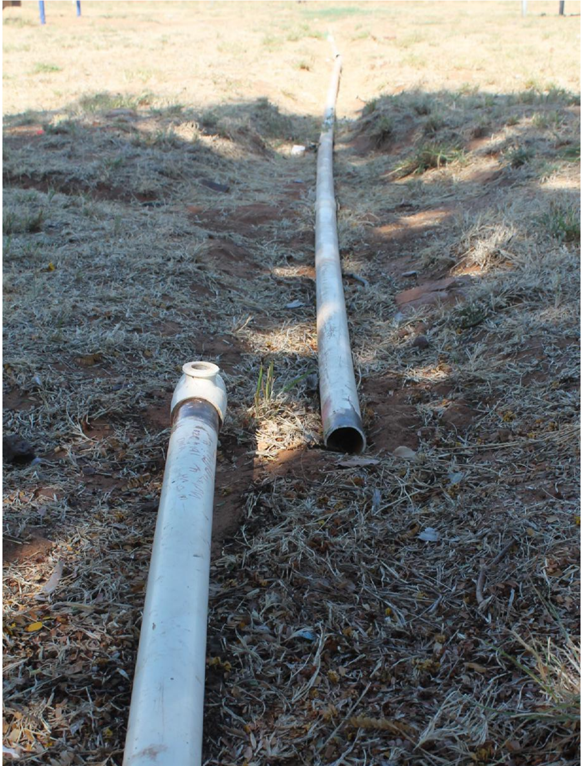
Figure 77: Abandoned and disconnected water pipes
