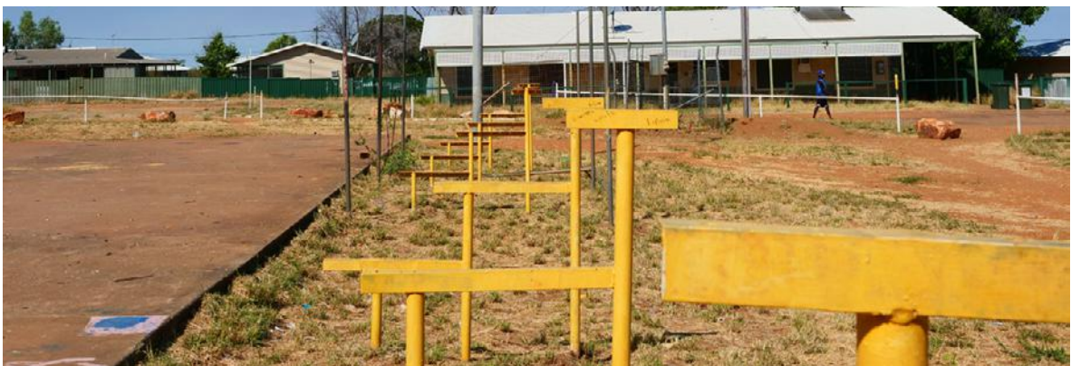
Figure 49: Condition of existing spectator seating
