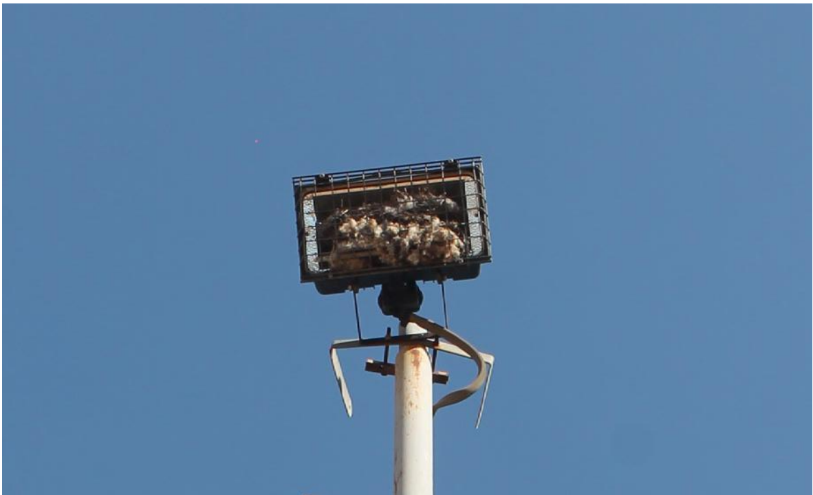
Figure 64: Existing floodlights are damaged and inoperable
