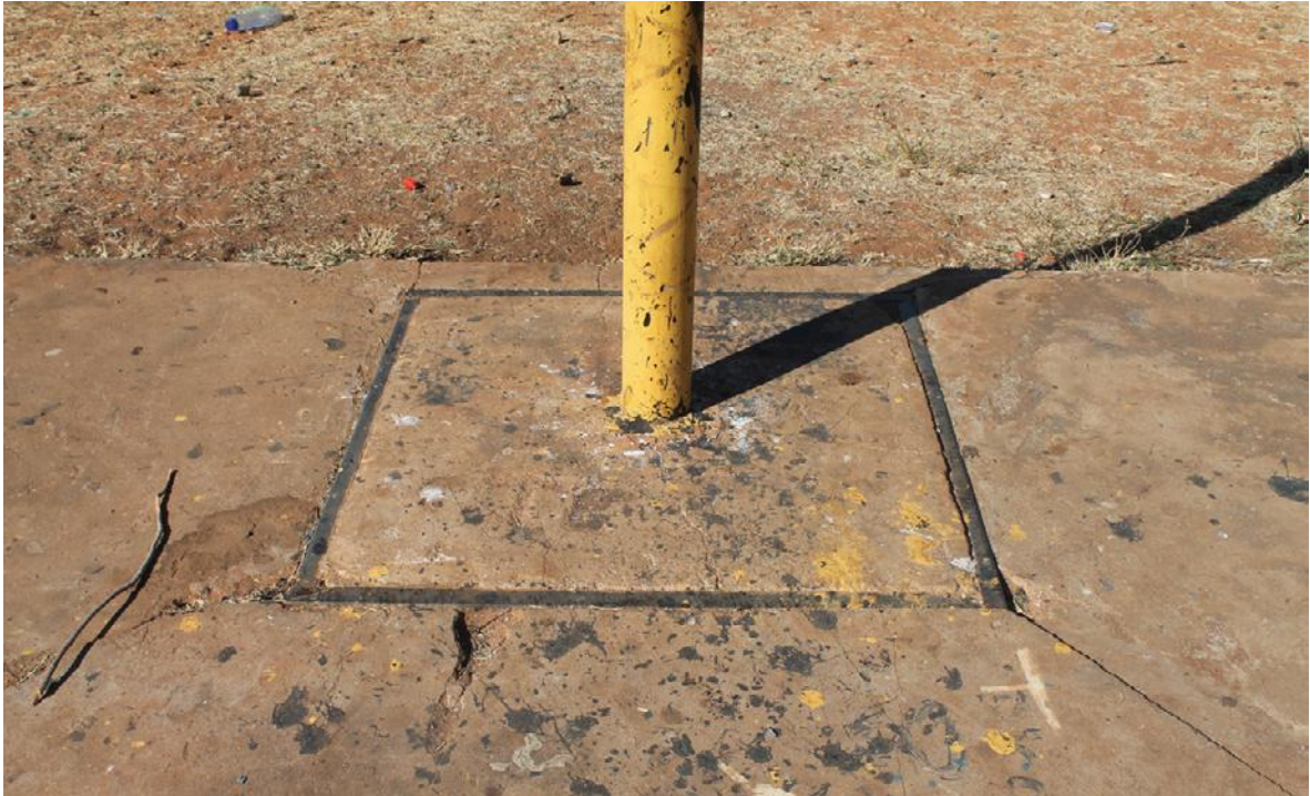
Figure 45: Base of hoop post
