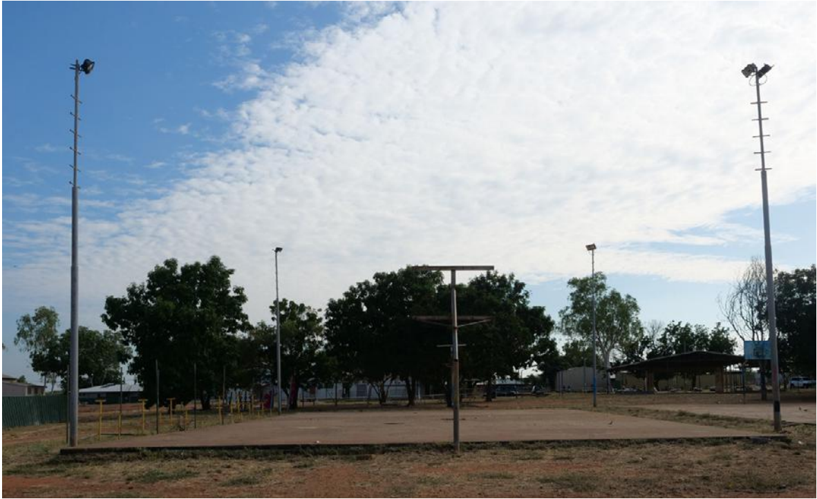
Figure 63: 8 floodlights and 6 posts - one on each corner of the courts
