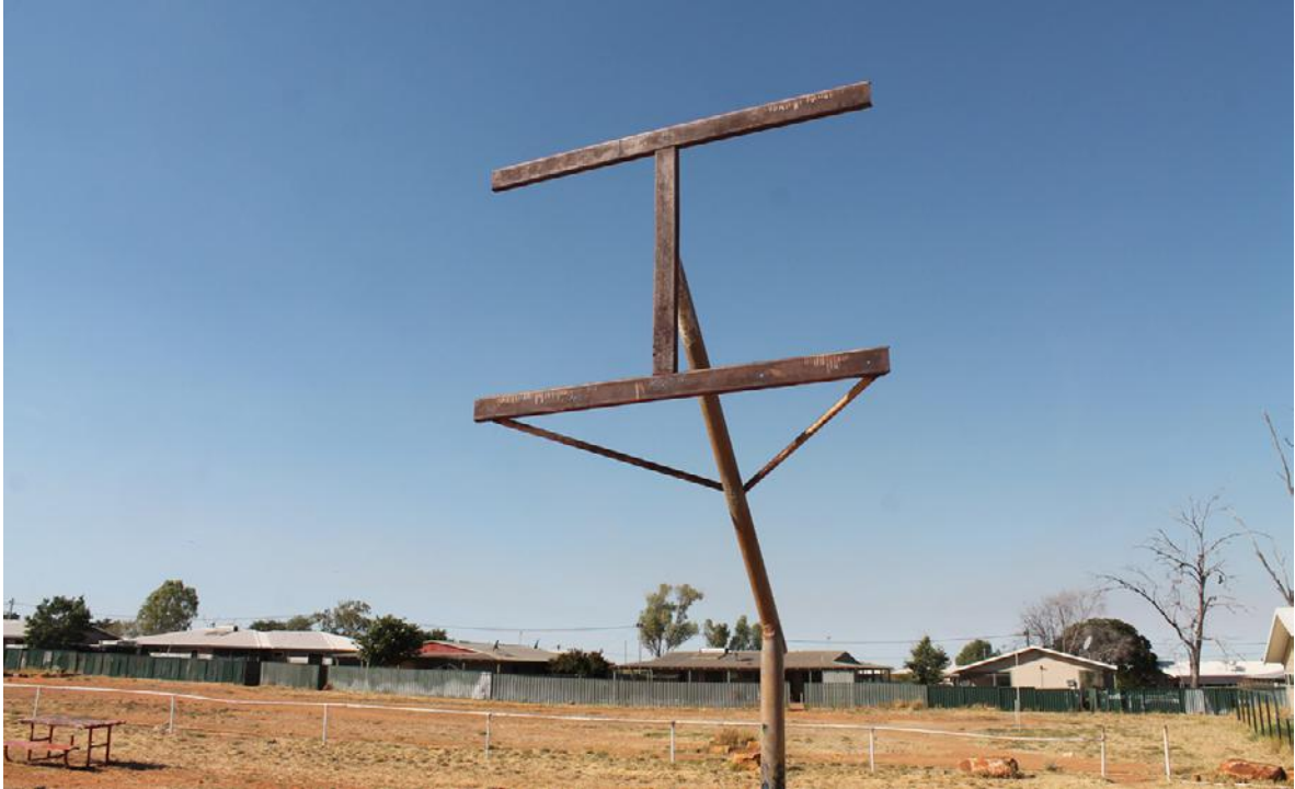
Figure 51: Condition of existing hoop - Court 2
