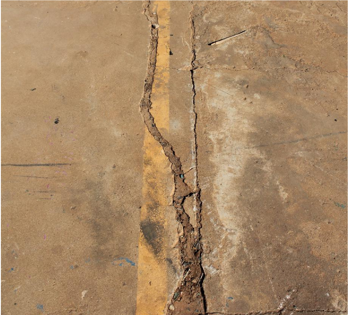
Figure 48: Cracks on court
