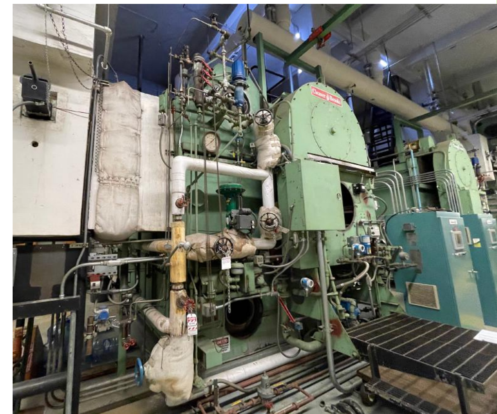
Image 3.3 (top right): Steam piping from Powerhouse to main campus.
