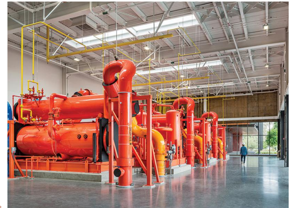
Image 7.9: Example: Hydronic heat pump plant at Stanford University.
