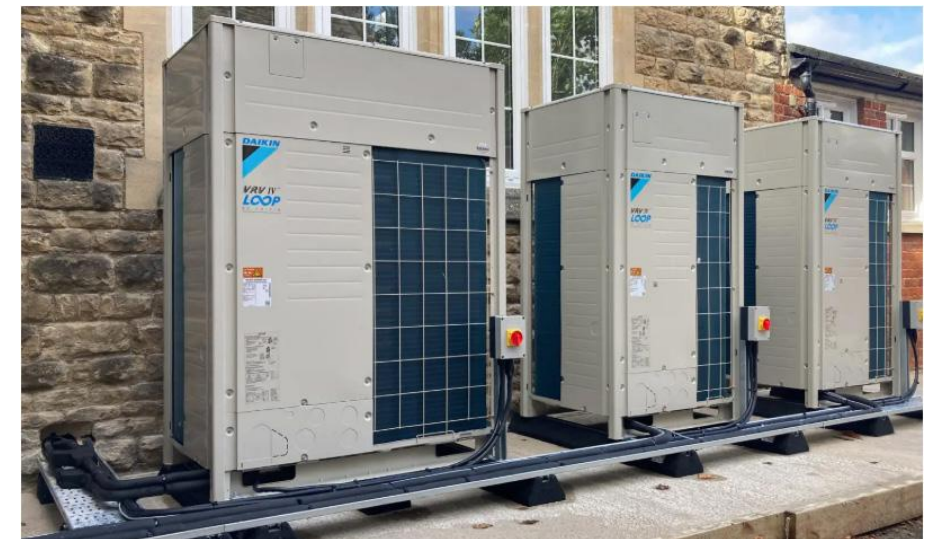
Image 7.14: Daikin VRF outdoor units.
