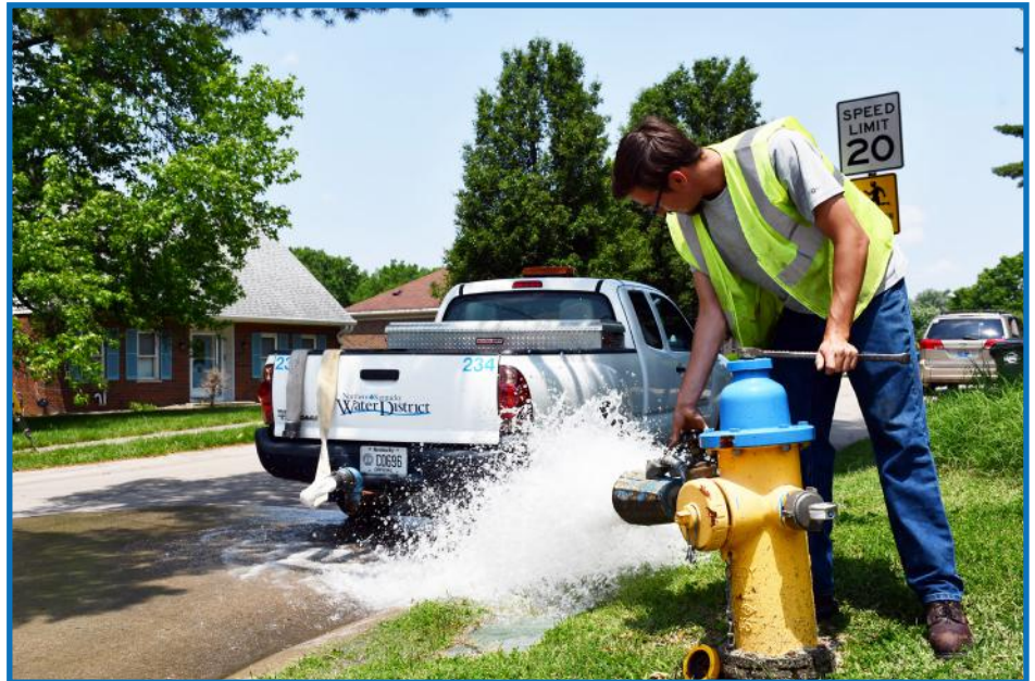
NKWD will either use a diffuser (pictured here) or a hose to control the waters path as it comes out of the hydrant.
