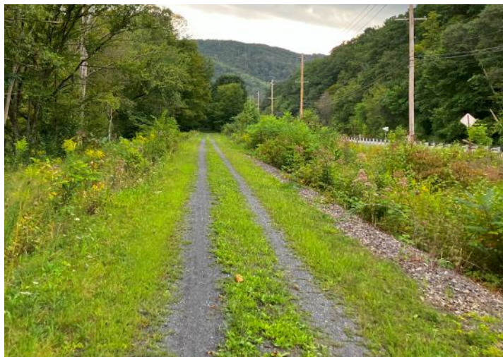
Above: Example of a crushed gravel trail in which grass has invaded the trail surface, both along the edges and in the center of the trail.
