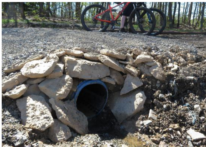
Above: The headwall of this culvert is also made up of natural rock. (Photo credit: Trail Association of the McKean/Elk Divide [TAMED].)
