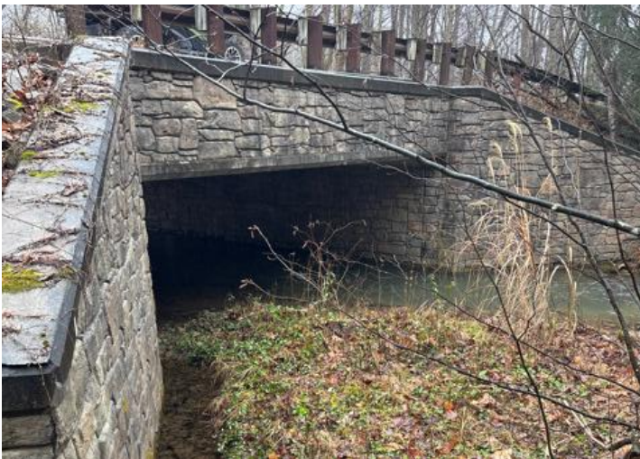
Above: A trail bridge on the Great Allegheny Passage crosses Ramcat Run, a tributary of the Youghiogheny River.
