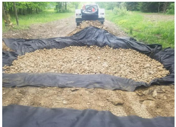
Above right: French mattresses allow water to pass through geotextile fabric while still supporting the trail’s foundation. (Photo credit: Cambria County Conservation District, Cambria County, PA.)
