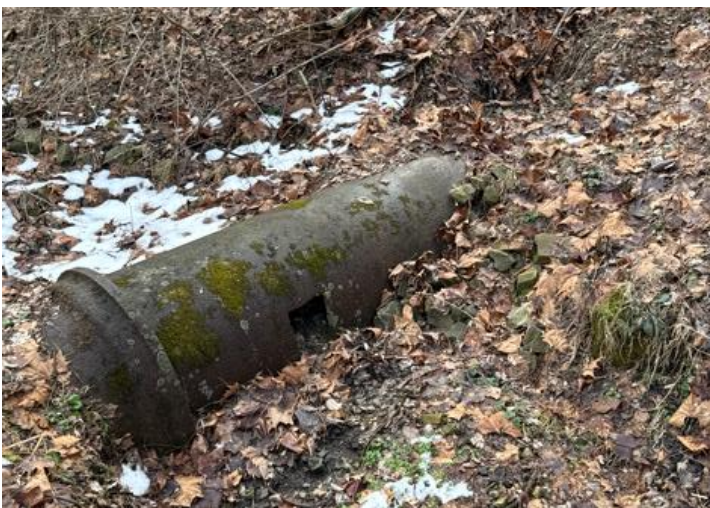
Above: The land around this old iron pipe has long shifted, and it is no longer functioning as intended. It also has a large hole in the side.
