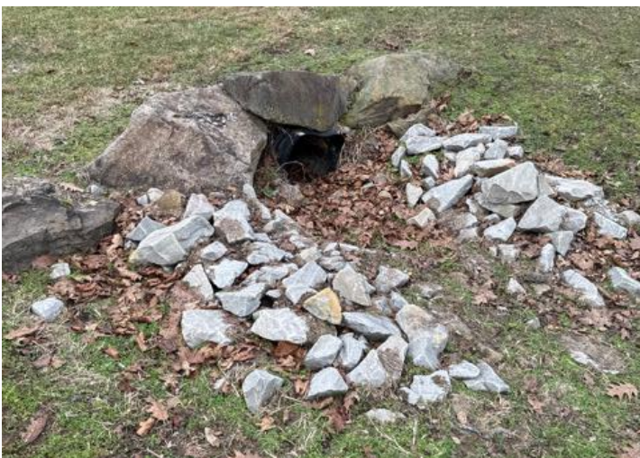
Above: The headwall and wingwalls of this culvert are made up of natural rocks and boulders.
