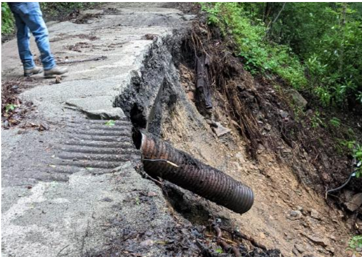
Above: A major landslide has rendered this small pipe, which was already under-capacity, inoperable.
