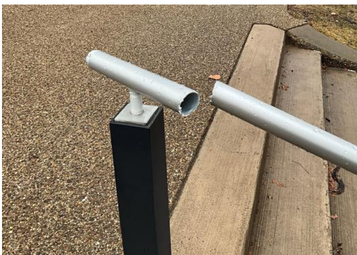
Above: This damaged safety railing on an urban trail should be repaired to prevent inadvertent injury to trail users.
