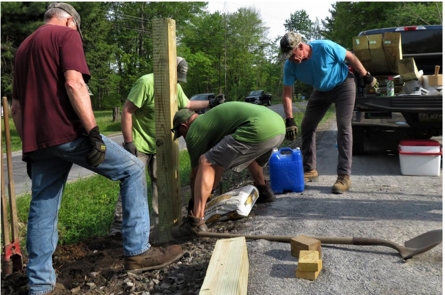
Above: Volunteers building a gate for Pennsylvania's Knox & Kane Rail Trail. (Photo credit: Trail Association of the McKean/Elk Divide.)
