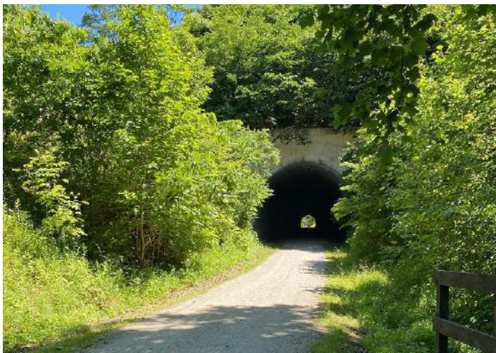
Above: The 849-foot-long Pinkerton Tunnel on the Great Allegheny Passage in Upper Turkeyfoot Township, Somerset County, PA.
