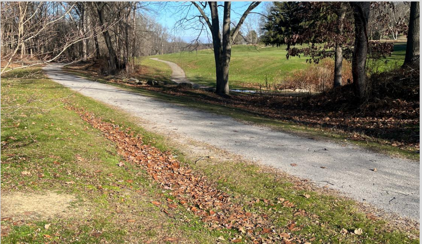
Top left: A swale hugging a cliffside along the Great Allegheny Passage in Perry Township, Fayette County, PA.
