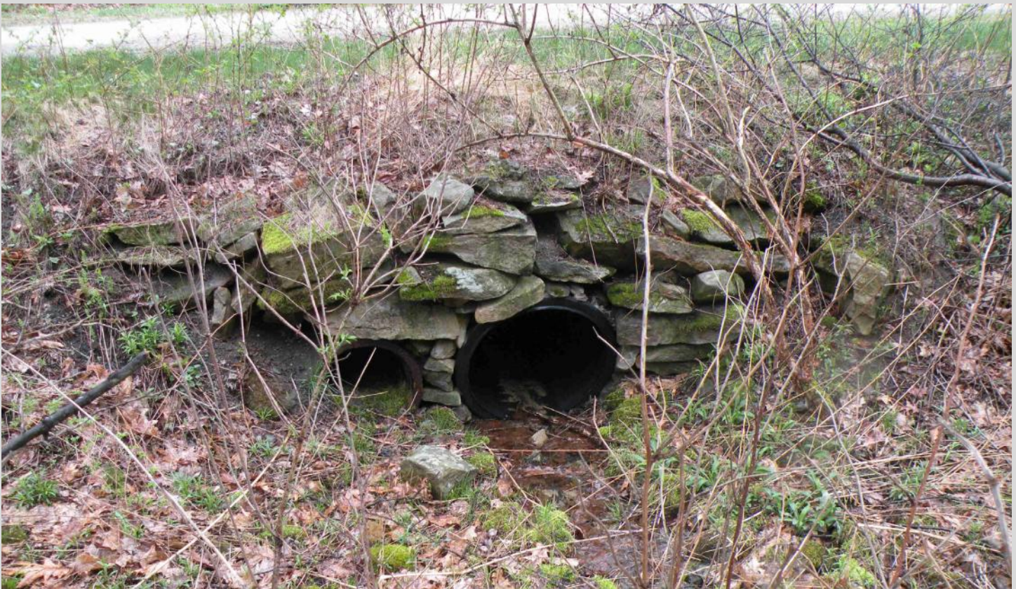
Top left: A trail organization volunteer inspects a concrete headwall and culvert serving Pennsylvania's Great Allegheny Passage.
