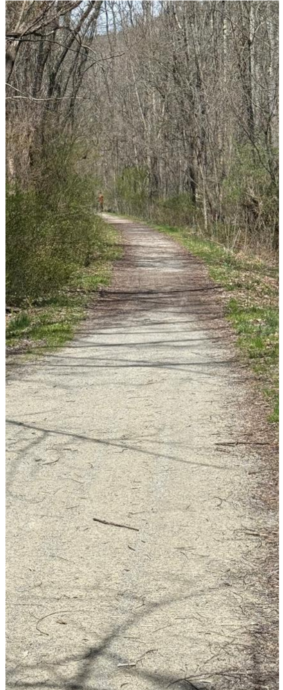
Above: This crushed gravel surface shows evidence of pooled water, indicative of a low point that has not been properly draining.
