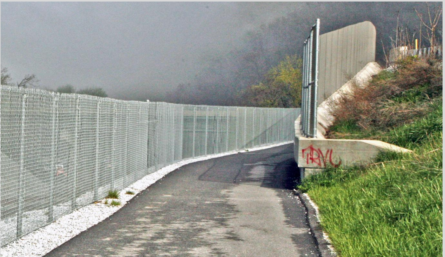
Top left: A cut stone block retaining wall along the Lackawanna River Heritage Trail in Scranton, PA.
