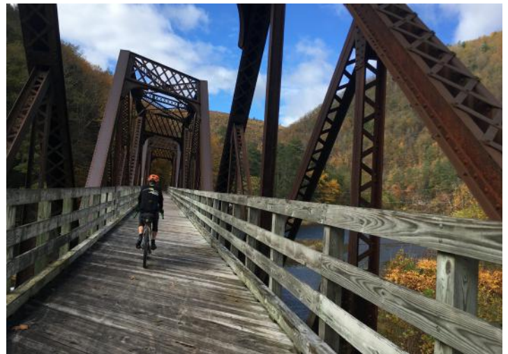
Above: A former railroad truss bridge repurposed for the Pine Creek Rail Trail in Watson Township, Lycoming County, PA.
