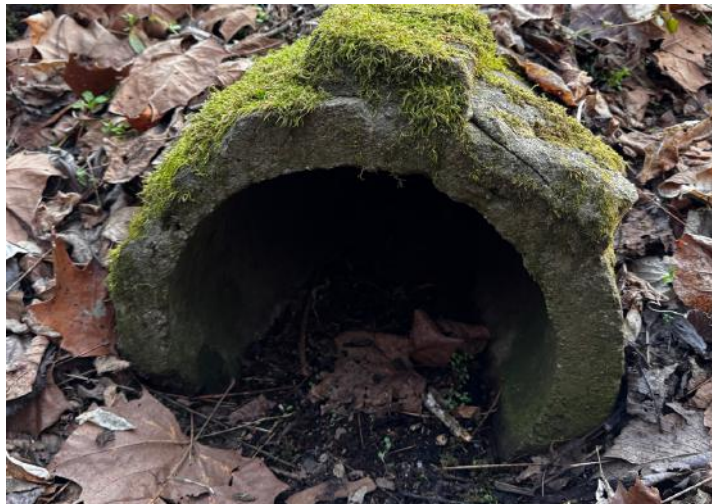
Above: Many concrete pipes along rail trails were originally constructed for the former railroads their rights-of-way once served.
