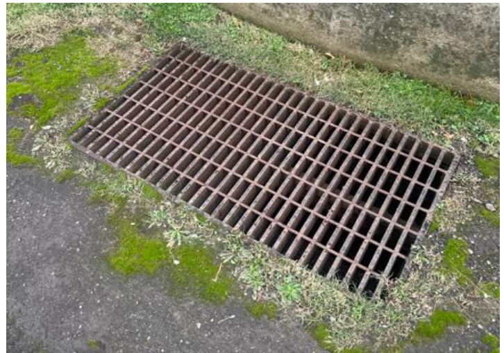
Above: Asphalt and concrete trails, which are usually impervious, often feature stormwater inlets covered by drainage grates.
