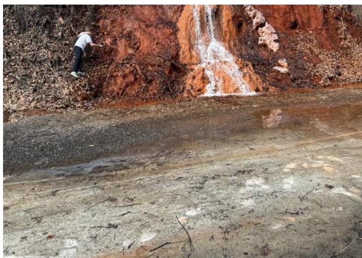
Above: The lack of a swale next to this crushed gravel trail means that the flow from this waterfall simply sheets across the trail surface.
