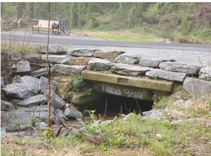
Above left: It may be surprising to see a concrete culvert from 1914 used on a modern trail, but this structure on Pennsylvania’s Northwest Lancaster County River Trail has stood the test of time.
