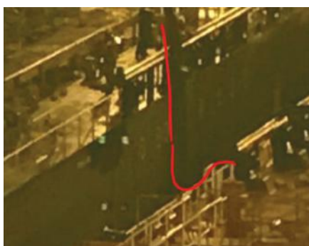
Incorrect lift causing U in hose
