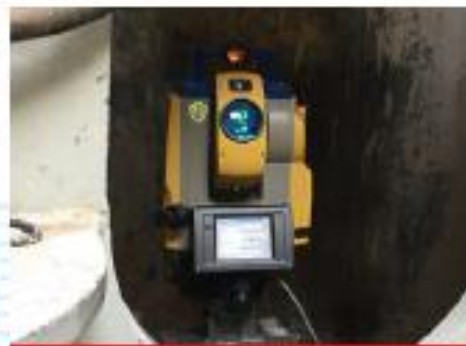
Shaft Station positioned behind the jacking frame thrust block in the launch shaft
