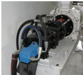
Main drive 250-500 HP electric motor and hydraulic pumps
