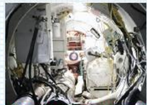
TGS 100 target is axially mounted behind the MTBM's articulation cylinders at line and grade, registers the position and angles of incidence of the red laser
