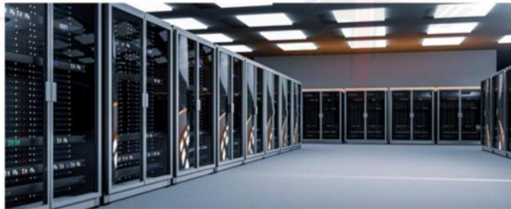
Fire extinguishing for server cabinet and computer bay
