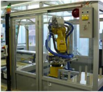
Fire extinguishing for equipment closed robotics
