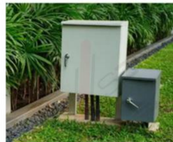
Fire extinguishing for outdoor electrical box
