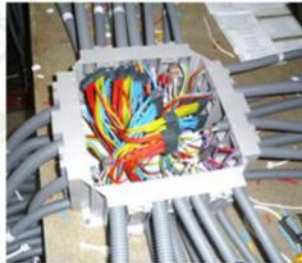
Fire extinguishing for junction box in attic
