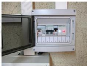
Fire extinguisher for spa electrical box
