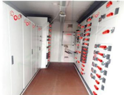
Fire extinguishing ship electrical room
