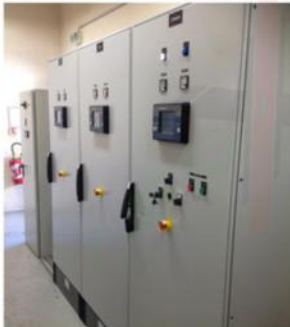
Fire extinguishing control cabinet
