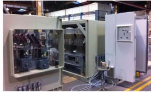
Fire extinguishing for automation and control cabinet
