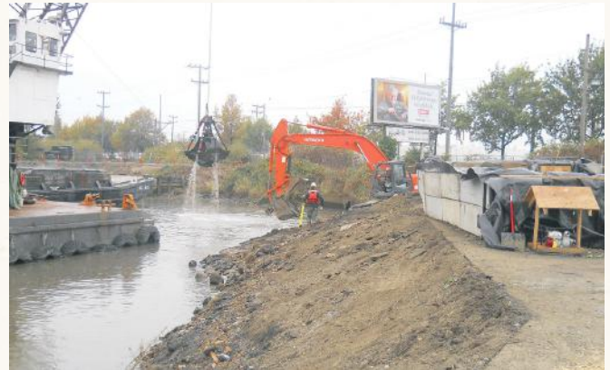
Excavation of contaminated sediment from the Lower dxʷdəw River Superfund site. Courtesy of the Seattle Municipal Archives, #169655, Series 7001-01.
