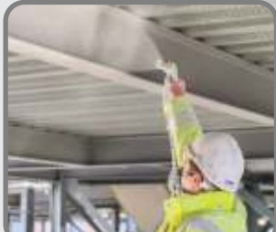
PASSIVE FIRE PROTECTION
