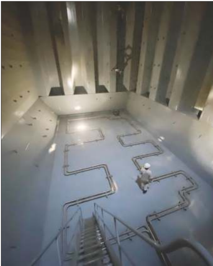
A cargo tank coated with MarineLINE® and has been in service for years.
