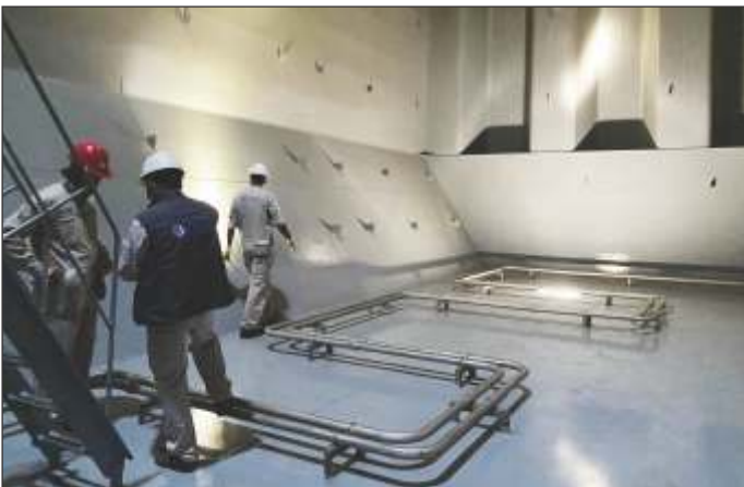
APC technical and inspection teams walking through a fully cured, completed cargo tank with MarineLINE®.
