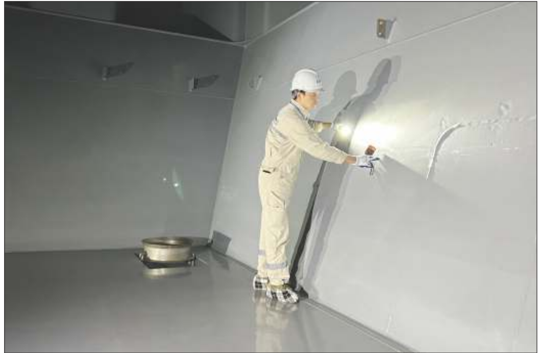
Inspection in progress to look for any pinholes in the coating that do not meet standards and marked to be repaired before final sign off on the cargo tank.
