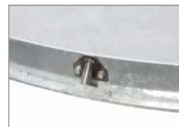
drainage stub pipes
