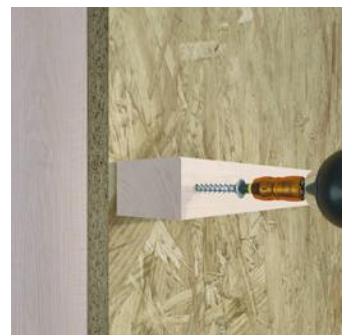
Mounting of installation level
