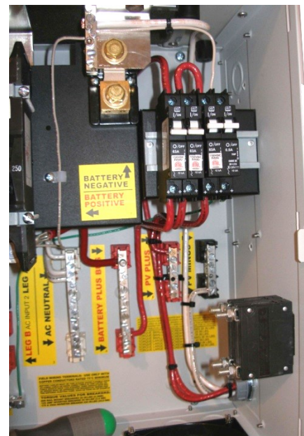
63 amp din rail DC-GFP wired with a 63 amp PV disconnect and a 63 amp controller output breaker.
