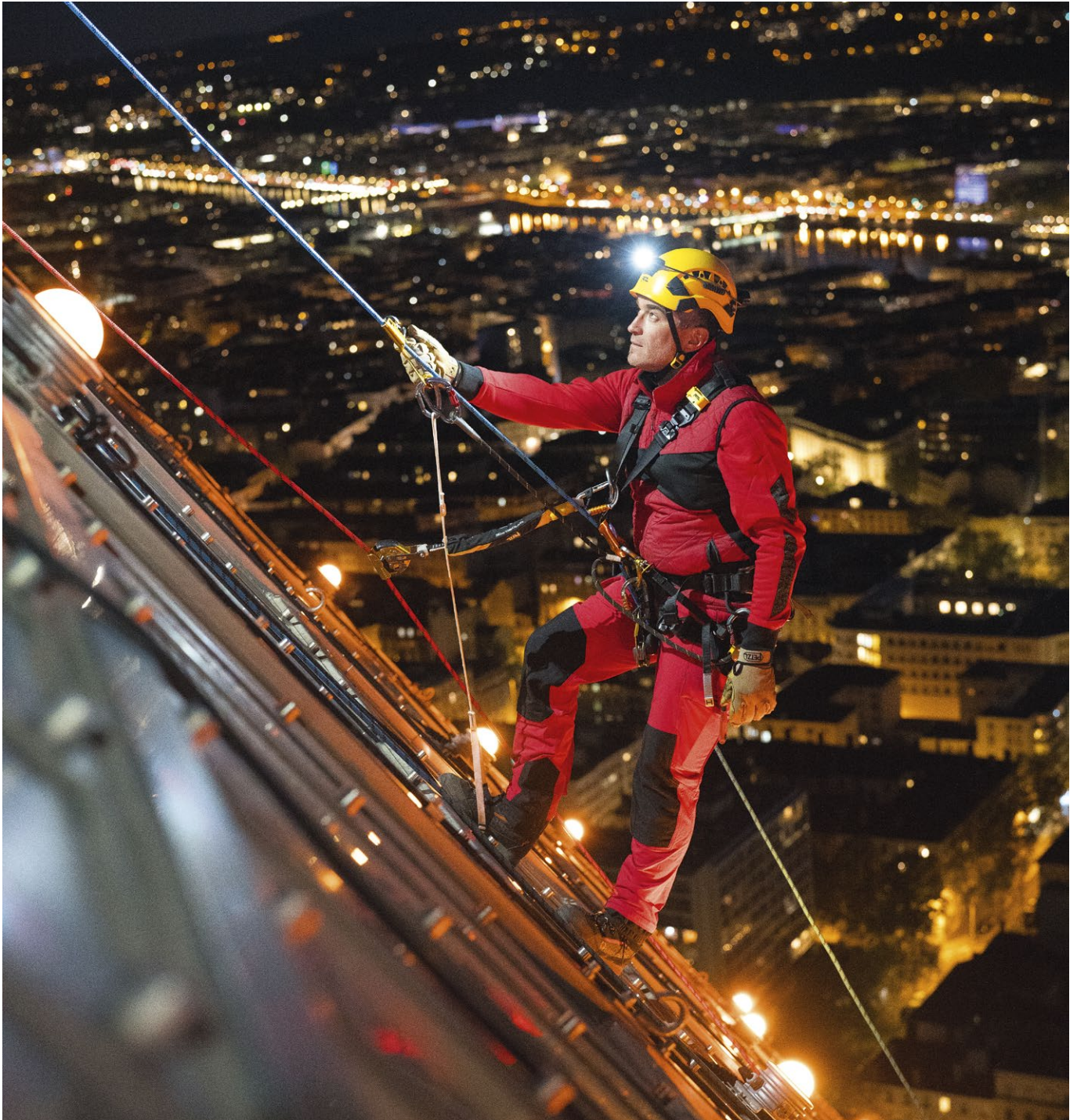
Glass window maintenance, Tour Crayon de la Part-Dieu, Lyon, France © 2024 Petzl Distribution - Lafouche - Bleu Ciel Services (BCS) - Tour Crayon de la Part-Dieu
