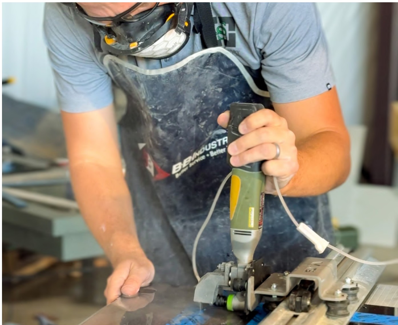
Cutting GPTP using a small angle grinder and a small-diameter cutting wheel with a water source eliminates dust. (Courtesy of Pasha Starykov, Star Tile & Stone, LLC)
