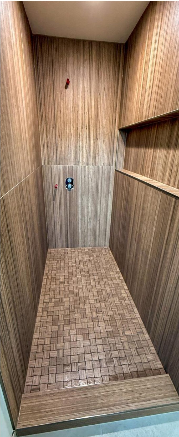
R&R Tile and Renovations installed this large-format 2'x4' wood-look tile with a basketweave mosaic and hidden tileable drain.
