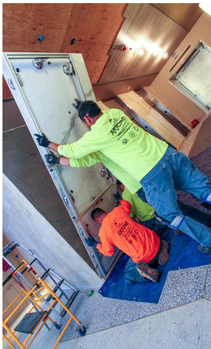
Installing GPTP on a commercial wall using a suction cup rack makes the job easier and safer. (Courtesy of Artcraft Granite, Marble, and Tile)
