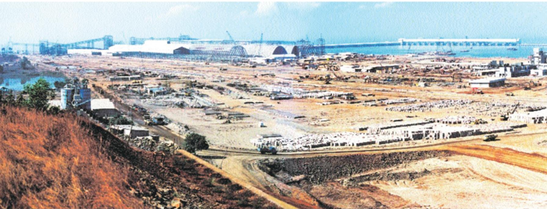
1. CONSTRUCTION OF THE BULK TERMINAL IS UNDERWAY IN 1988. VISIBLE ARE THREE LARGE SHEDS FOR STORAGE OF FERTILIZERS, ORE, AND FOOD GRAIN, IN THE EARLY STAGES OF CONSTRUCTION
