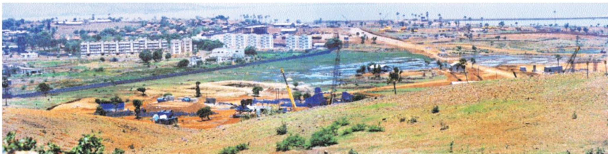
L. STONE-CRUSHING PLANT ATOP SHEVA HILL, DURING CONSTRUCTION IN 1995. DEFENCE BUILDINGS ARE SEEN IN THE BACKDROP
