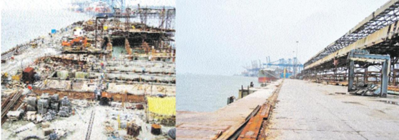
DEMOLITION OF THE BULK TERMINAL WAS CONSIDERED A NATURAL OUTCOME OF THE SUCCESSFUL PUBLIC-PRIVATE PARTNERSHIP MODEL.
