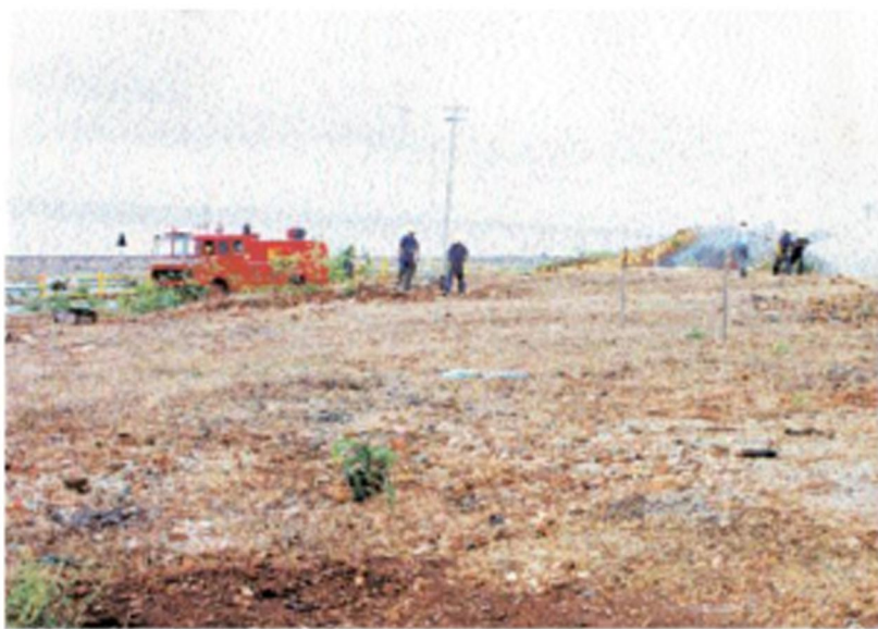
ENGINEERS INSPECT SHEVA HILL, WHERE THE PORT ADMINISTRATION BUILDING NOW STANDS, IN THE EARLY STAGES OF CONSTRUCTION
