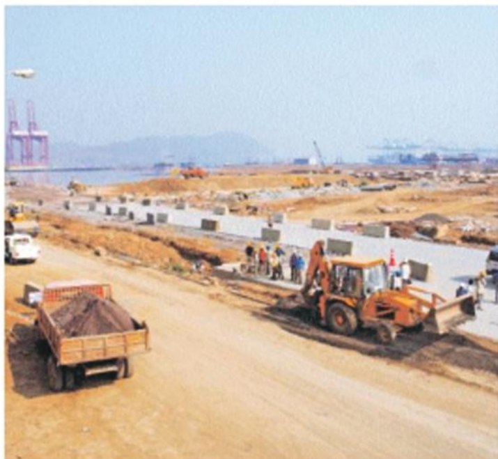
THE BULK TERMINAL BEING DEMOLISHED TO MAKE WAY FOR A NEW CONTAINER TERMINAL.
