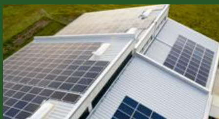
ON SITE SOLAR PANELS
