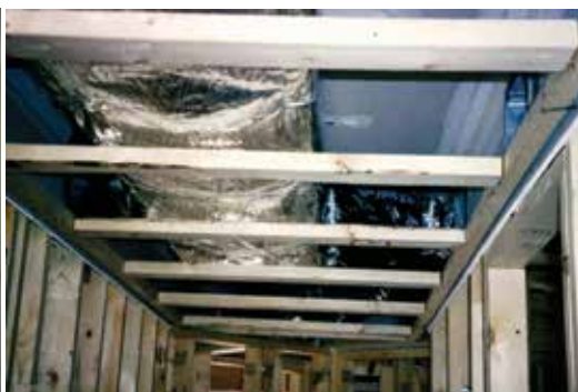
Photograph 8: Dropped Ceiling – Ductwork located in a hallway/corridor dropped ceiling. The supply and returns are in the same dropped ceiling.
