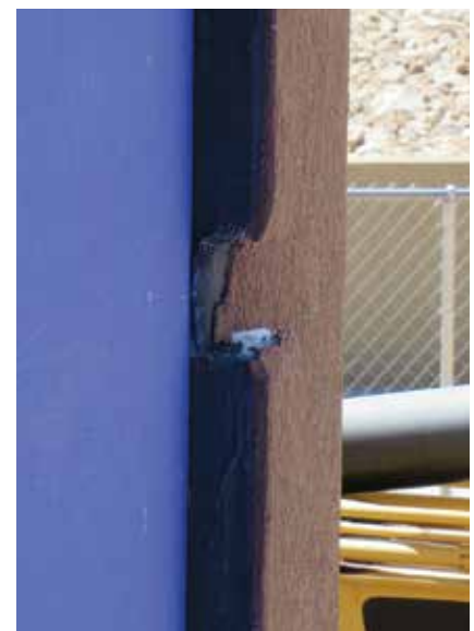
Figure 4: Damage along the inner edge of the EIFS-clad wall panel from strapping.
