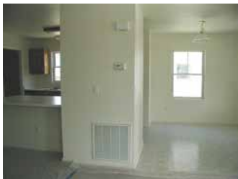
Photograph 7: Single Return – The single return at the main floor level has an "offset" to handle blower noise.
