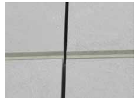
Figure 3: The vertical gap between wall panels is irregular at the four-way panel intersection due to excessive buildup of material at adjacent panel corners.
