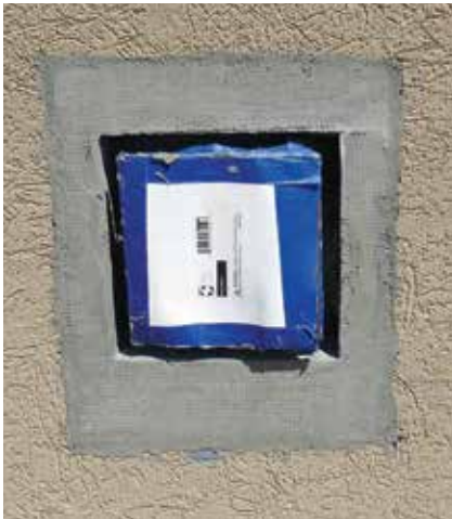
Figure 9: In-progress field repair of a field penetration. The size of the repair area is considerably larger than the size of the penetration itself.
