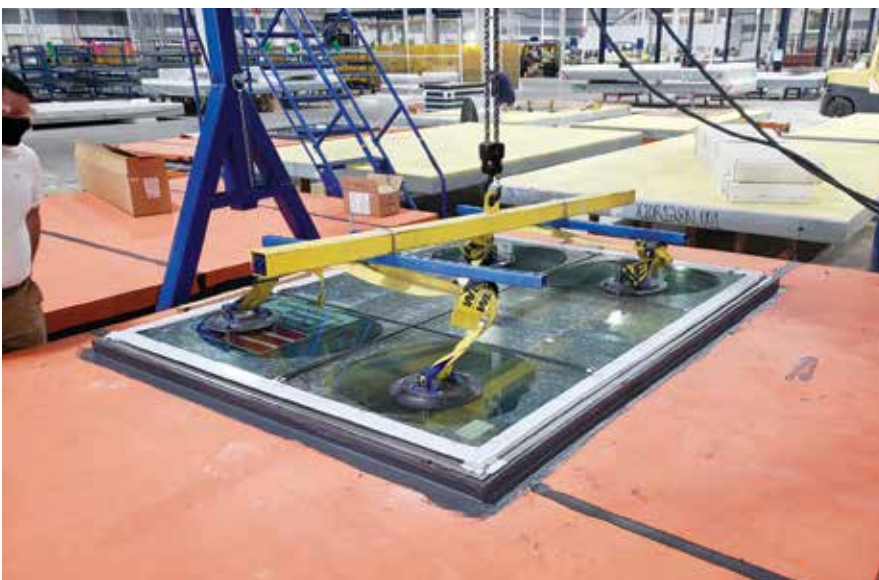
Figure 6: The punched window system is installed onto pre-treated wood bucks in the panel opening. This process is done entirely in the shop. The panel is shipped to the site with the cladding and fenestrations pre-installed.
