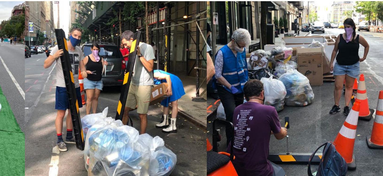
▲ The Open Plans Team together with CHEKPEDS build trash corrals in Hells Kitchen. July 2021
