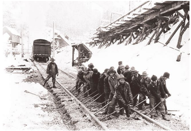
Photograph of Chinese American railway workers straightening track in the construction of the Cascade Tunnel ca. 1928.
