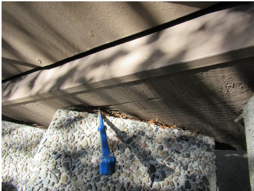
Figure 58. Decay damage pocket at exposed stair stringer.
