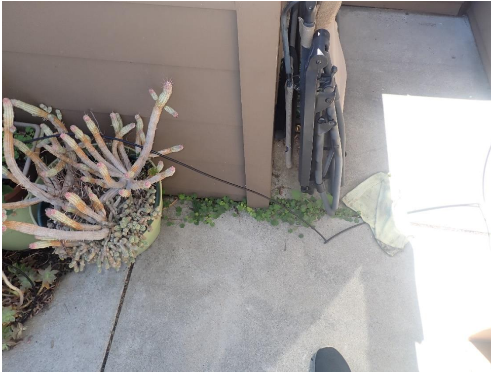
Figure 22. Growth on topping slab.
