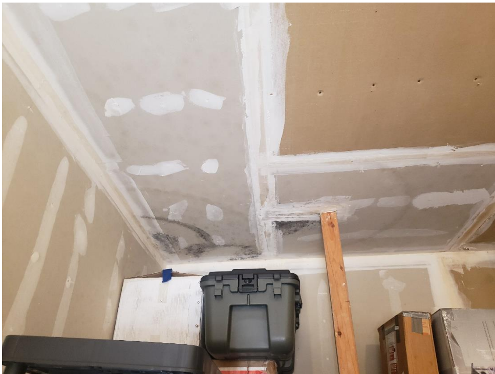
Figure 48. Bio growth on garage ceiling at active leak.
