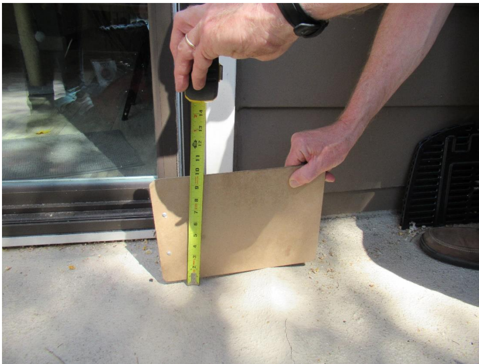
Figure 32. Hump in exposed waterproofing at 816 Wharfside (Building 2).
