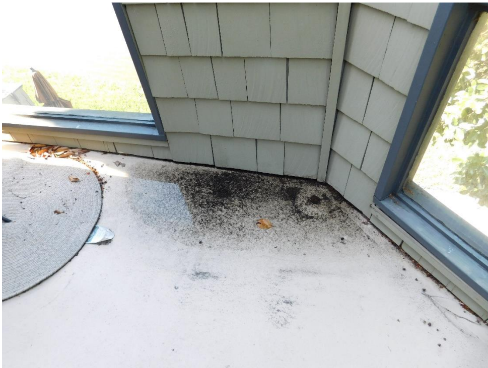
Figure 23. Ponding water at drain location.
