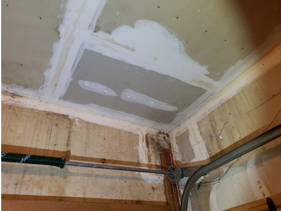
Figure 49. Garage walls and ceiling with water staining on both older and newer gypboard.
