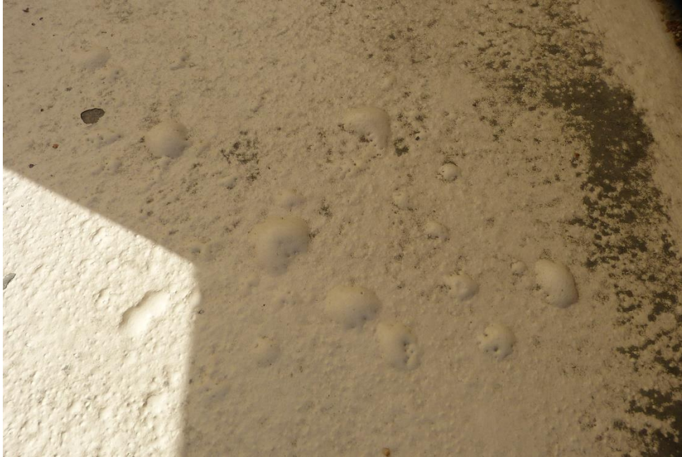
Figure 20. Distress to overcoating on exposed waterproofing.
