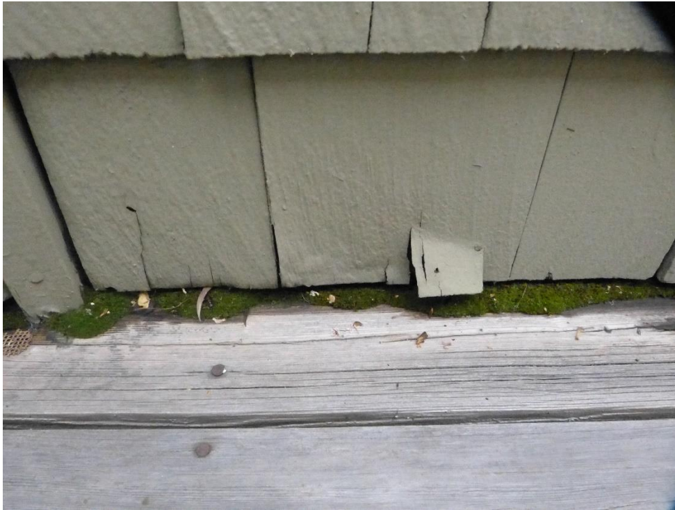
Figure 41. Bio growth on deck boards.
