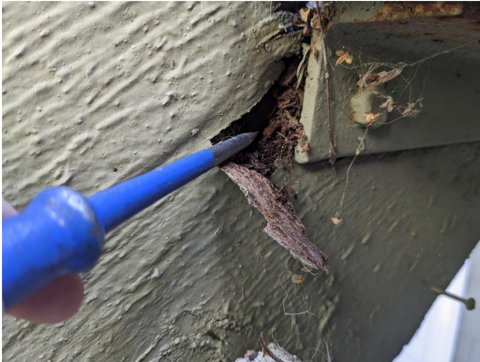
Figure 59. Decay damage at stringer support connection.
