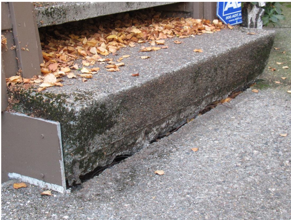
Figure 60. Base of entry stair with tall stair riser and gap between lowest riser and surrounding flatwork.
