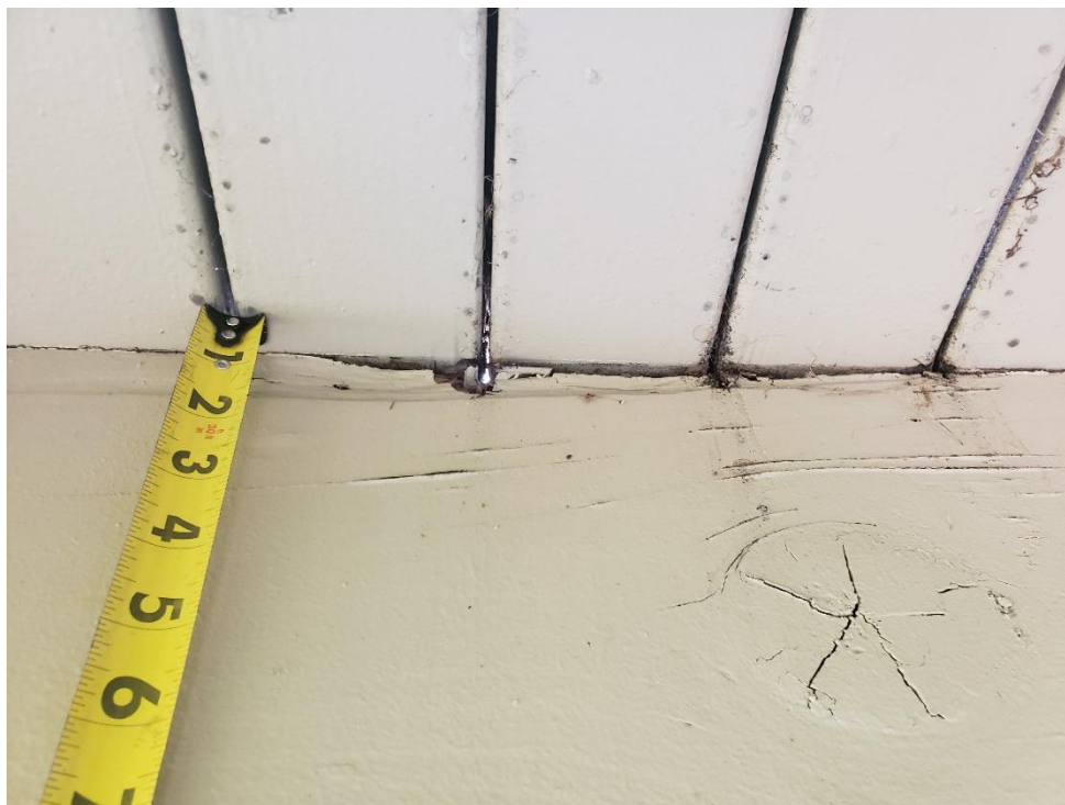
Figure 36. Localized wood decay at top of exposed joist.
