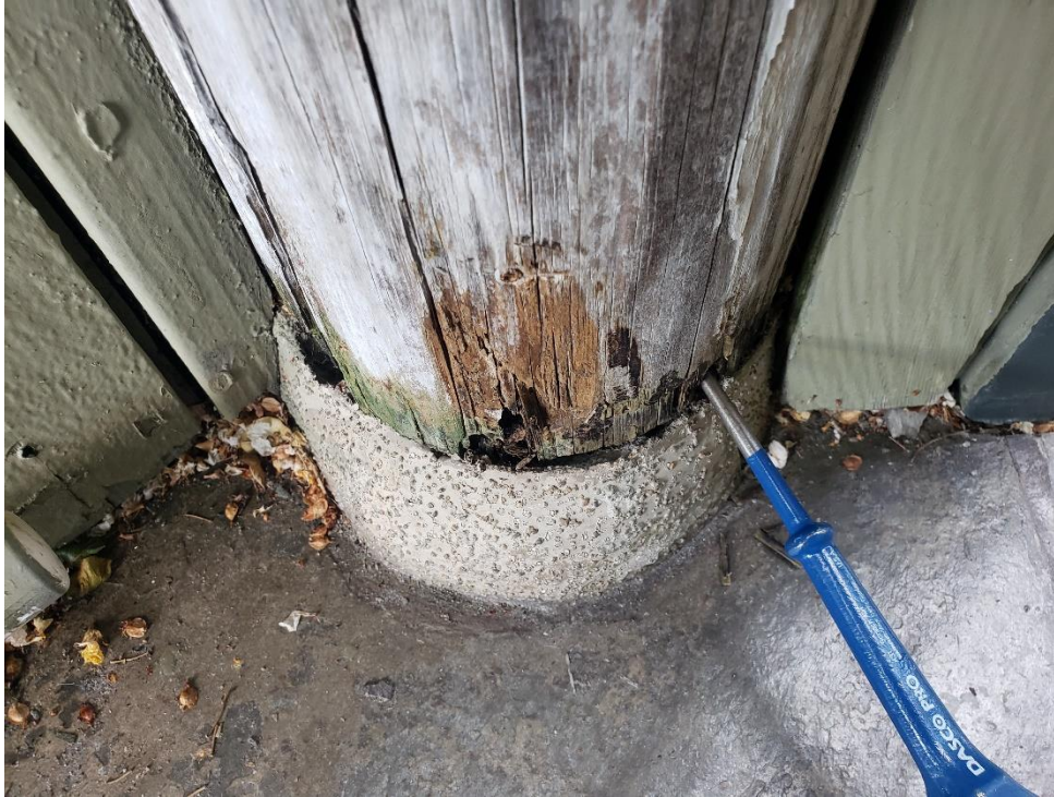
Figure 26. Decay damage at bottom of log post.
