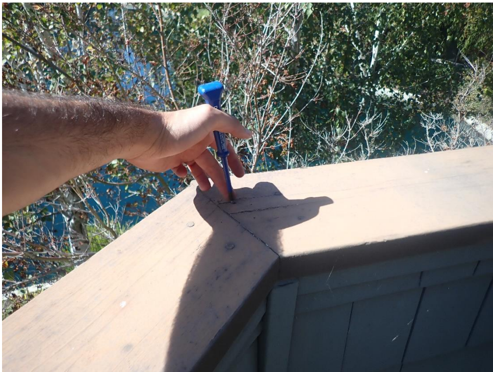
Figure 29. Decay damage in other guardrail framing.
