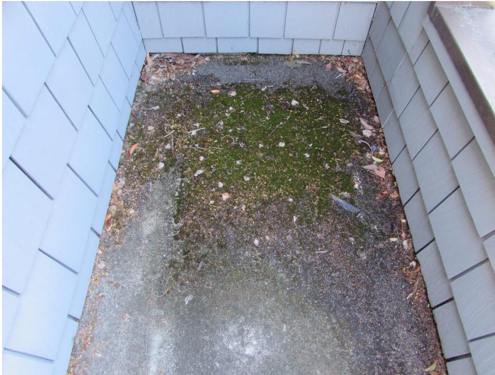
Figure 47. Bio growth on exposed topping slab.
