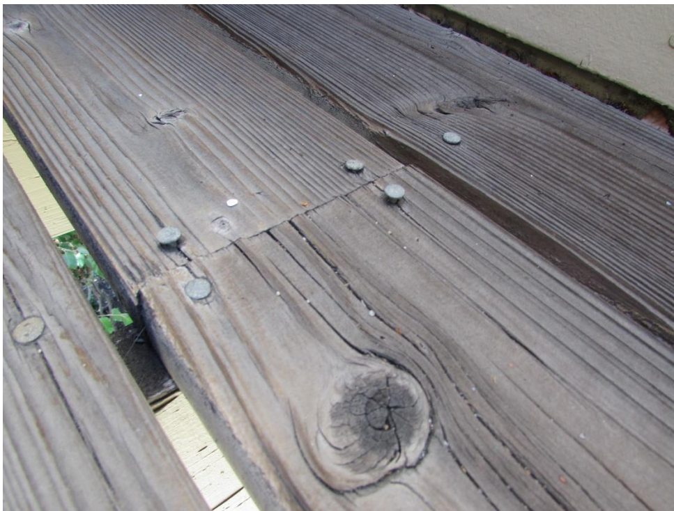
Figure 40. Deteriorated deck boards with nail popping.
