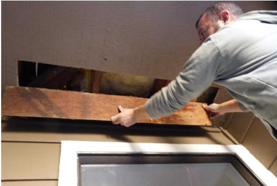
Figure 31. Water intrusion at local decay damage at 941 Shoreline (Building 26).
