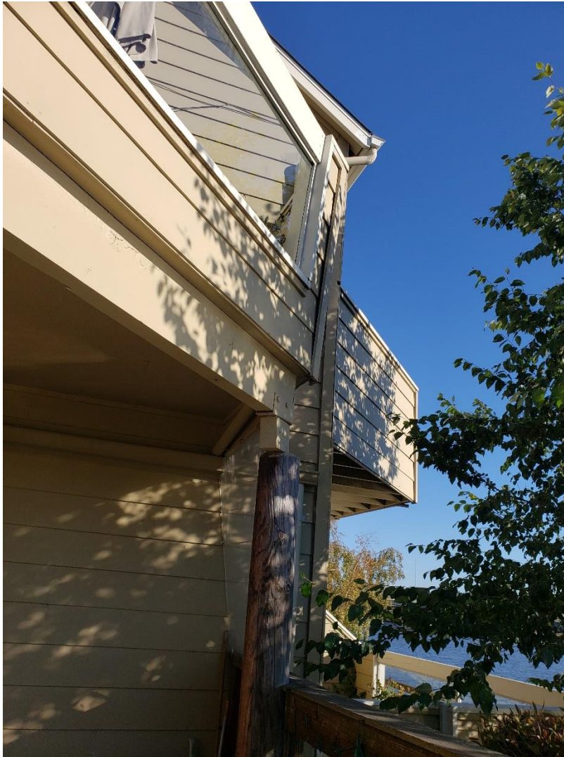
Figure 30. Leaning deck guardrail at 1130 Shoreline (Building 15).
