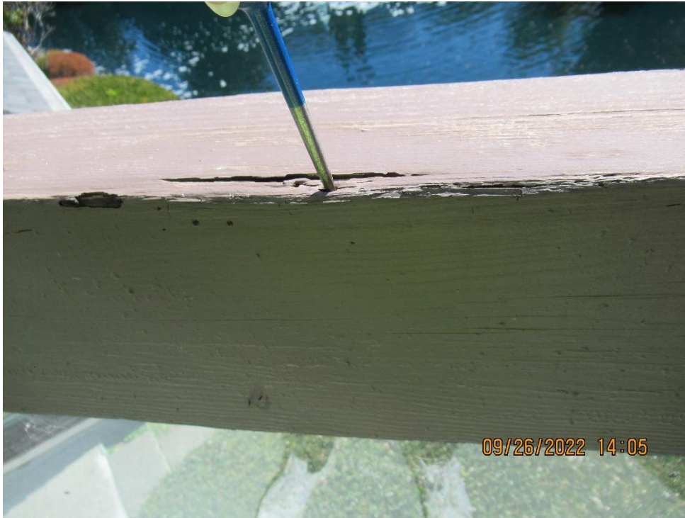
Figure 28. Decay damage in guardrail top rail.
