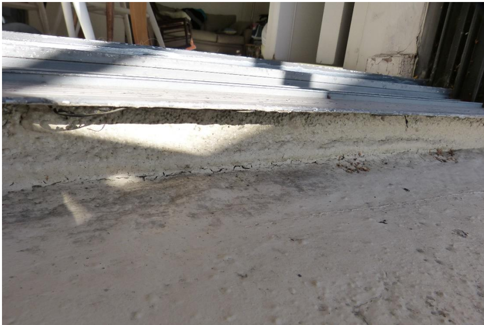
Figure 21. Cracking in upturned edge of exposed waterproofing.
