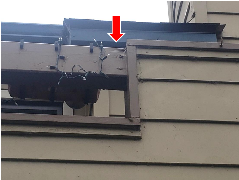
Figure 42. Decay damage to guardrail top rail.
