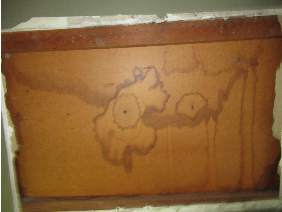
Figure 14. Inspection opening in ceiling of garbage and recycle area, showing moderate water staining.
