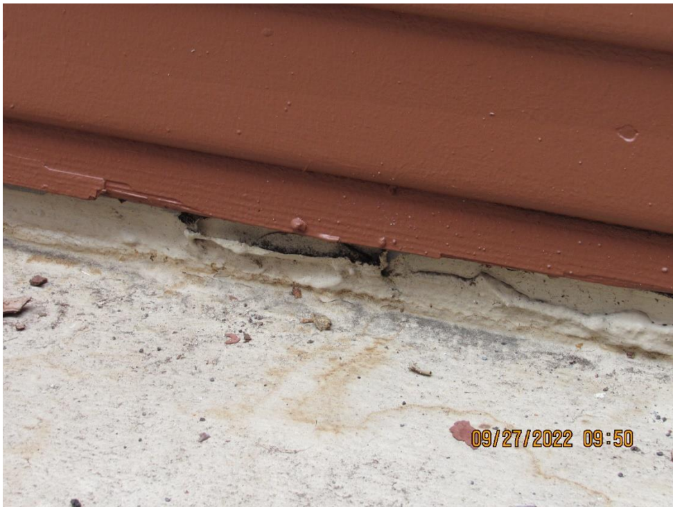
Figure 46. Peeling and cracking of exposed waterproofing at upturned edge.
