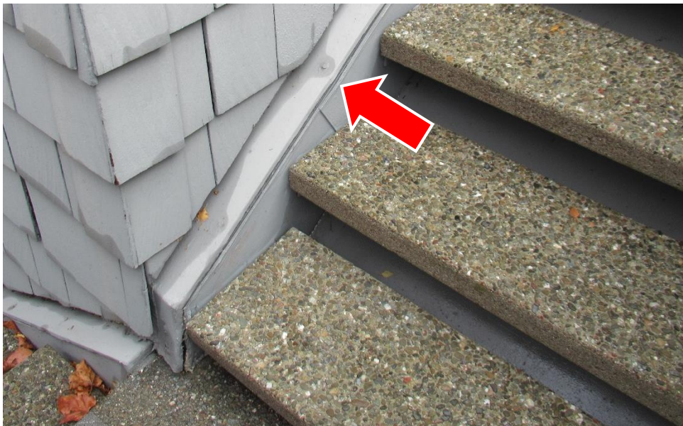
Figure 54. Stringer cladding out of position, allowing water intrusion.
