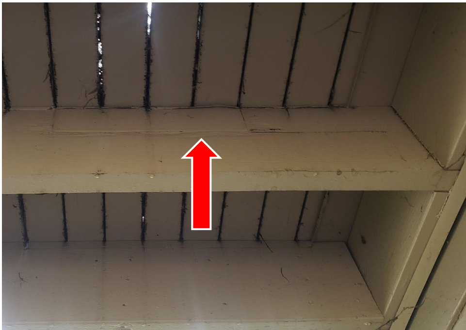
Figure 38. Inappropriate deck joist repair that compromises deck strength. Joist has been cut out and patched back in.
