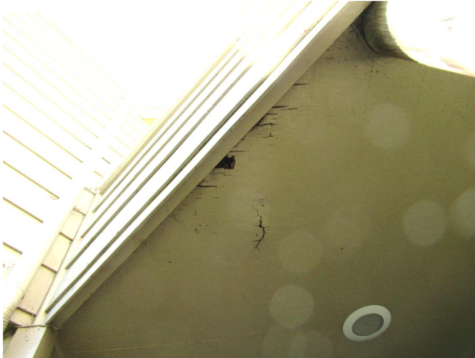
Figure 57. Entry deck soffit with decay damage.
