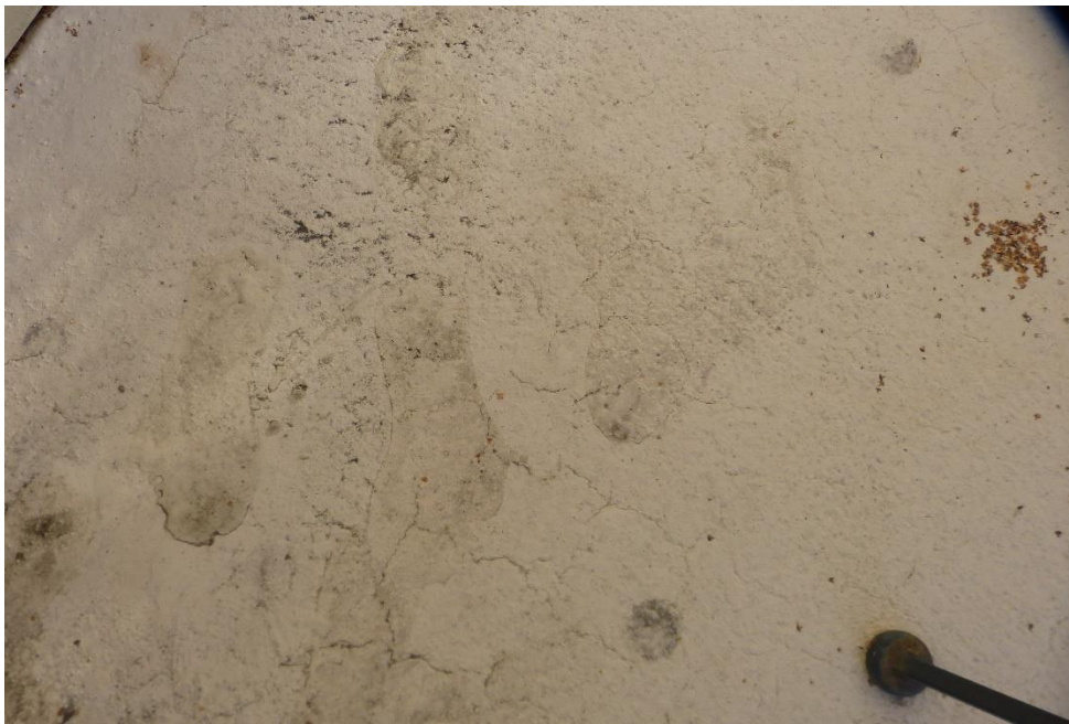
Figure 19. Distress to overcoating on exposed waterproofing.
