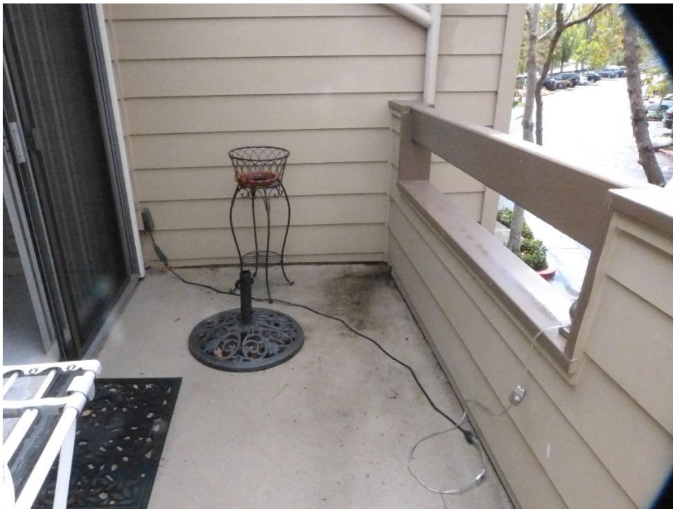
Figure 44. Unit deck above garage with exposed waterproofing.
