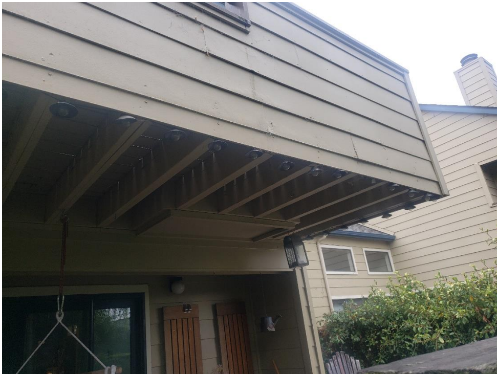
Figure 6. Unit deck not over garage with exposed framing.
