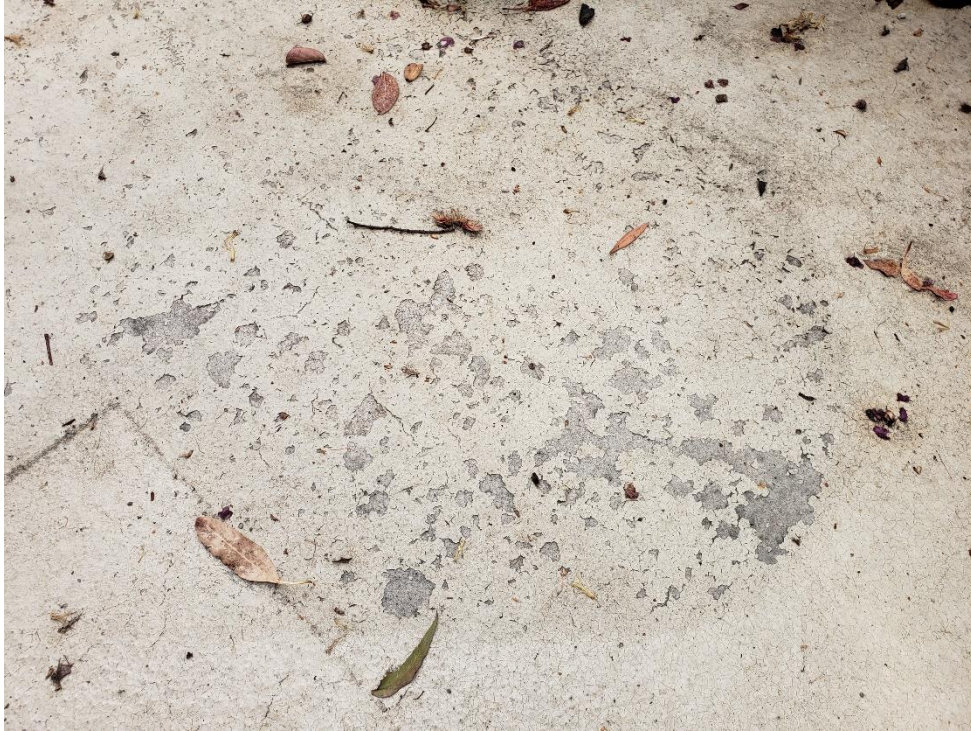
Figure 45. Bubbling and peeling of exposed waterproofing.
