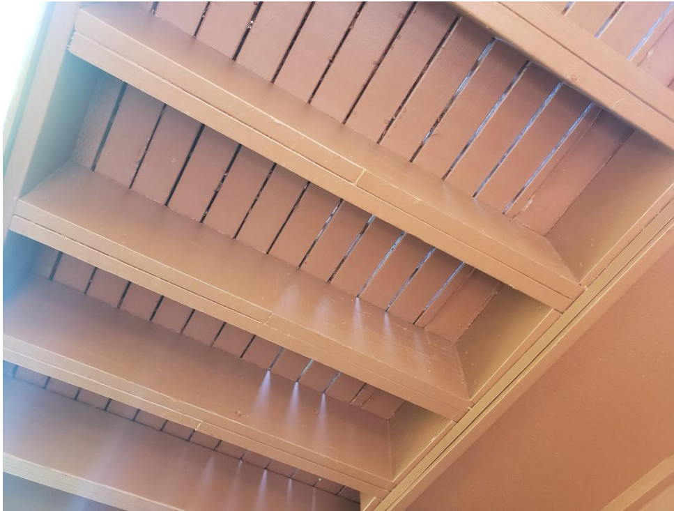
Figure 39. Inappropriate deck repair where joists have been cut back and then sistered.
