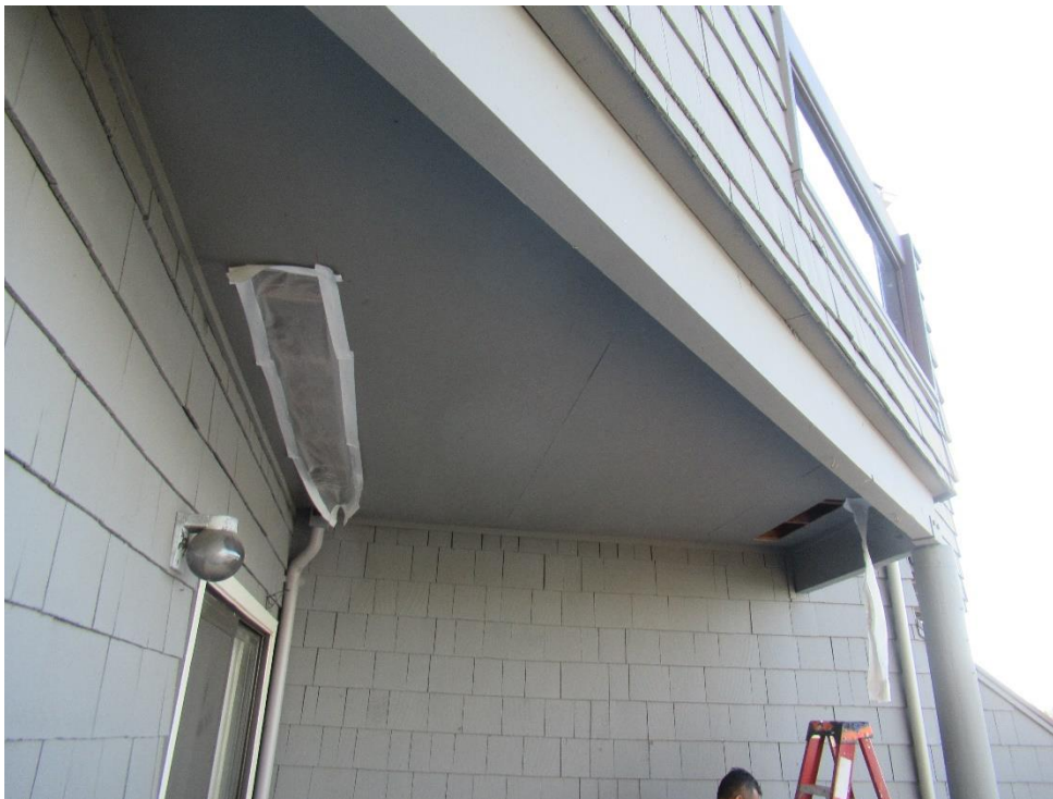
Figure 11. Inspection openings at unit deck not over garage with concealed framing.
