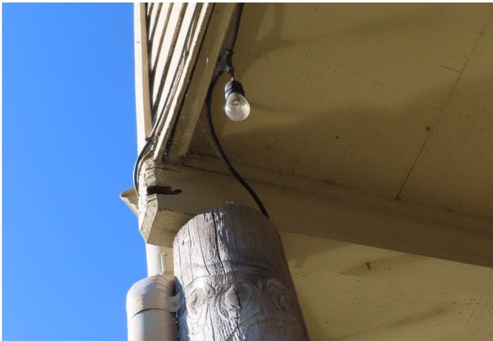
Figure 27. Decay damage in end of beam at 1088 Shoreline (building 13).
