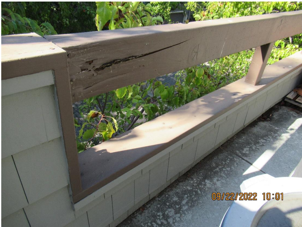
Figure 50. Decay damage to guardrail top rail.
