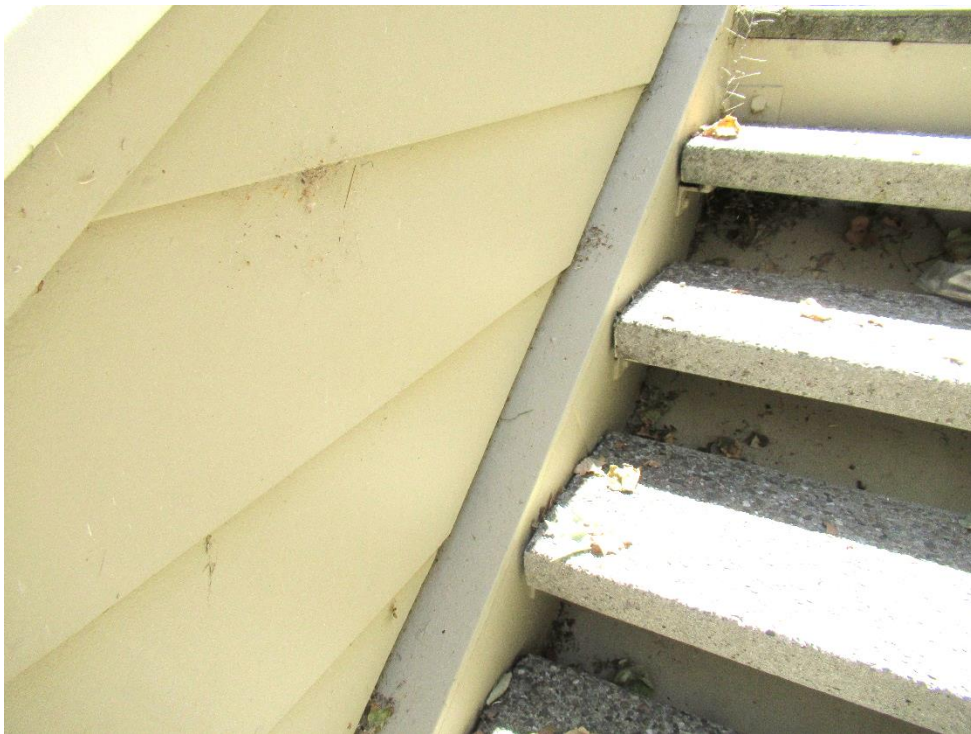
Figure 52. Street-side building stair with cladding on stair stringer and below treads.
