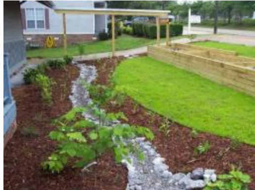
Bioswales help mitigate flooding by directing the water downhill and are used in place of traditional concrete gutters.
