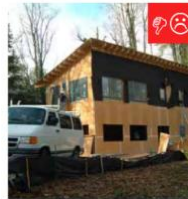
The building felt is not installed on the entire house.
