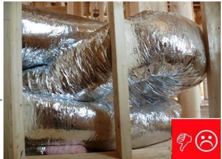
No excessive bends in flex ducts
