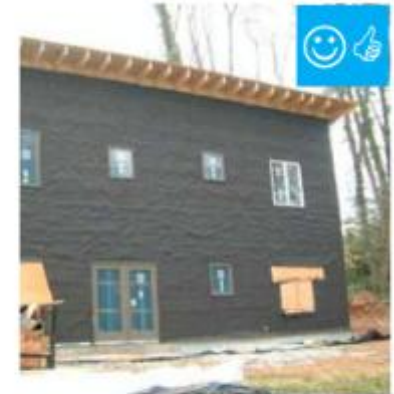
The building felt is installed on all exterior walls and provides a complete drainage system.
