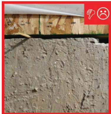
Un-sealed sill plates
