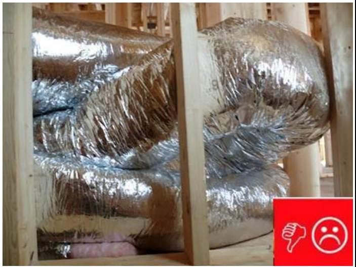
No excessive bends in flex ducts
