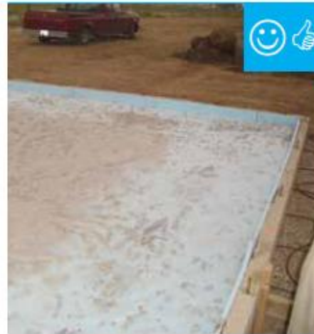
There is a polyethylene sheeting installed to provide a capillary break between the ground and slab.
