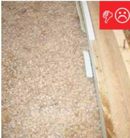
There is no polyethylene sheeting installed between the ground and the slab.
