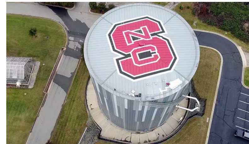
A thermal storage energy tank on the Centennial Campus of North Carolina State University in Raleigh.
