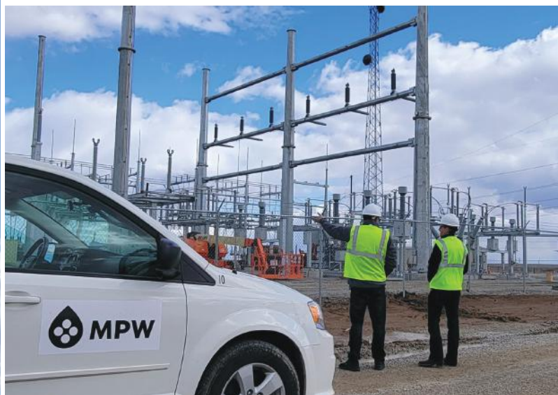
Massive steel poles, like the one shown at left carry Line 106 cross-country from MPW's West Substation to the new North Substation along Highway 38 (above).
