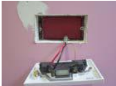
FireSure® Gasket installed ready for fire test. Note the box is not installed completely within the plasterboard and the gaps around the edge before testing.
