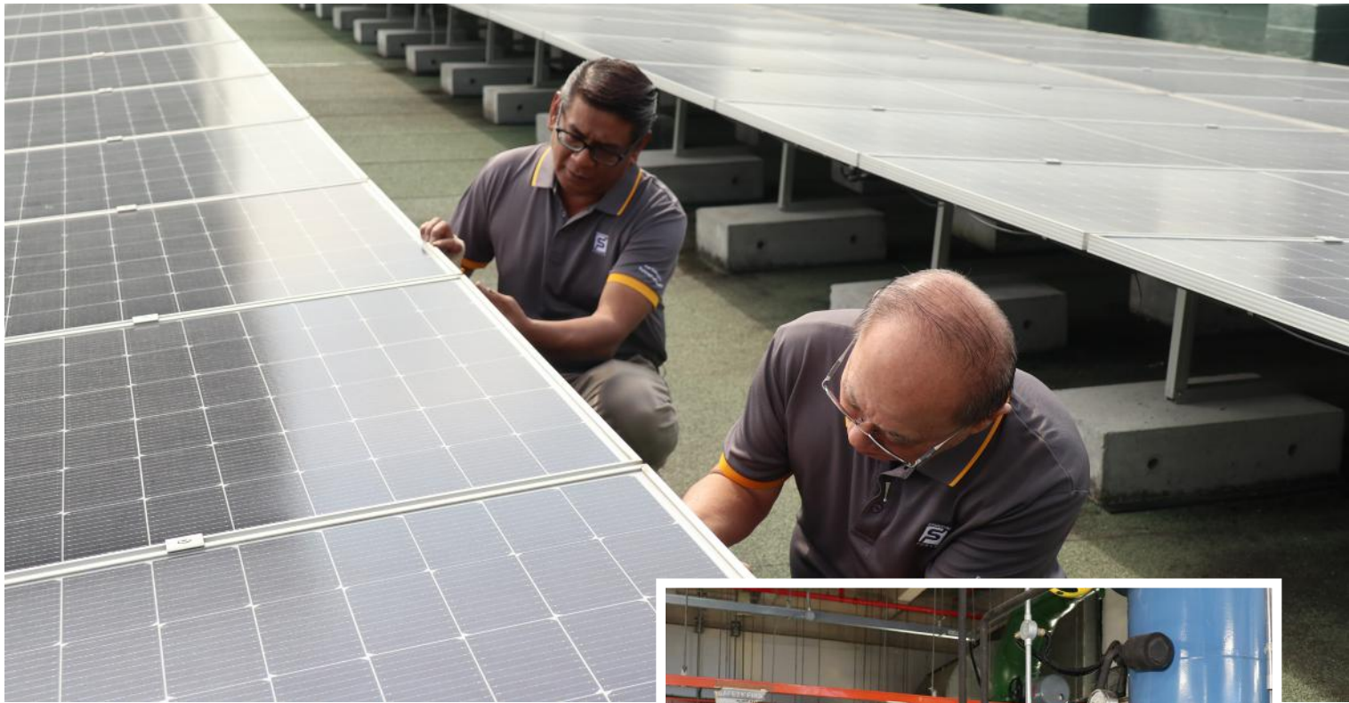
Photovoltaics installed on Singapore Pool's rooftop harnesses solar energy to power the building's passenger lifts and an entire office floor.
