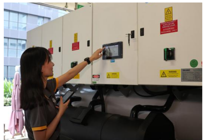
Engineers monitoring the refreshed chiller system to ensure optimal performance energy standards.
