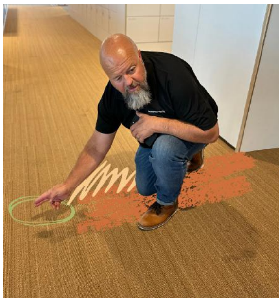
Colin Saddington inspecting adhesive stains
