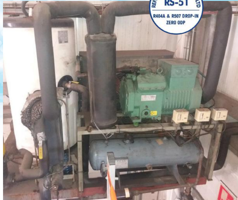
Refrigeration system formerly operating with R507 retrofitted to RS-51 (R470B)
