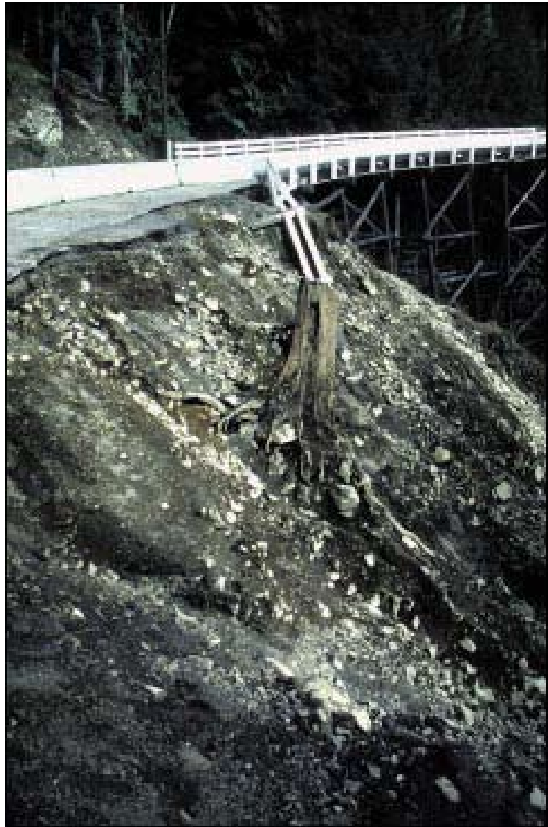
Figure 4.4-6 February 1996 SR-165 Bridge along Carbon River Landslide
