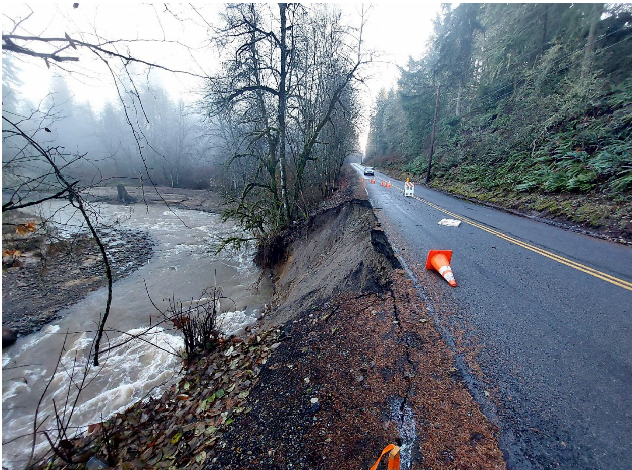
Figure 4.4-4 December 2023 Landslide on Johns Road East along Wilkeson Creek
