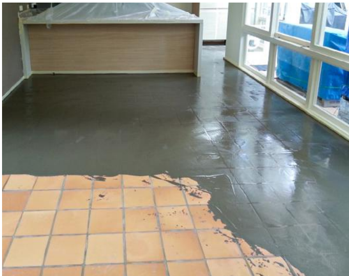
On a properly prepared tile floor, troweled-on patch can flatten the substrate to ready it for new tile.
