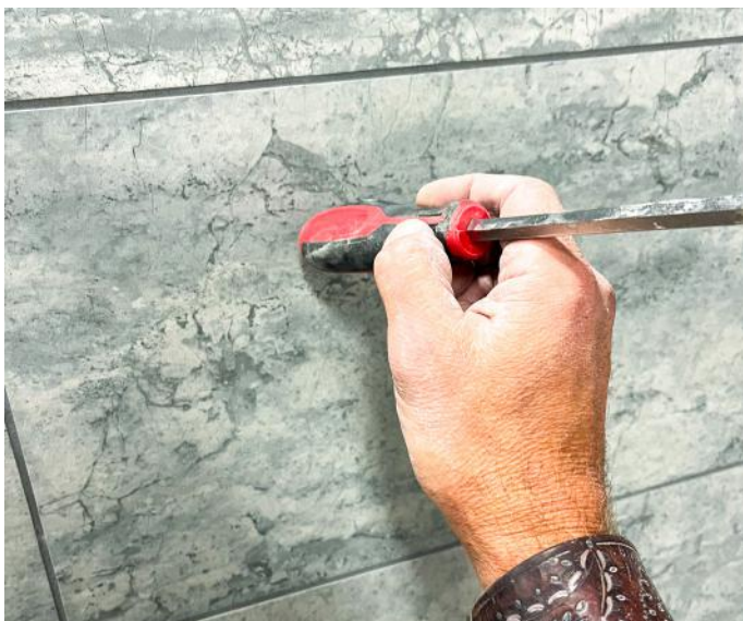
Tapping on the surface of the tile can reveal unbonded tile. Alternatively, it could be a membrane that yields a different tone. Photo courtesy of Dragonfly Tile & Stone Works, Inc.
