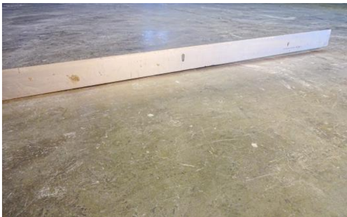
A 10' straightedge reveals a large low spot on a concrete floor.
