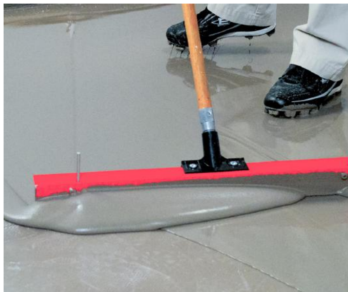
A Flowable Hydraulic Cement Underlayment (FHCU) applied over the appropriate primer can provide an acceptably flat floor.
