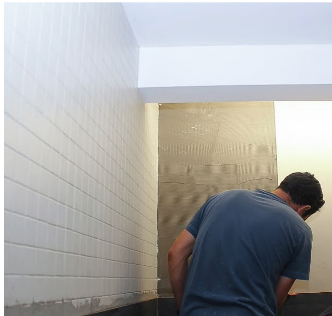
Rather than removing the existing tile, proper prep work allows for a tile-over-tile installation when utilizing the manufacturer’s recommendations.
