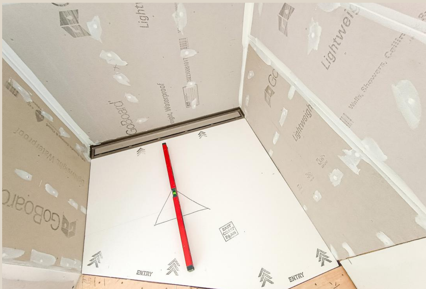
The master bath linear drain was installed into the Rapid Recess Blind Pipe Connector (BPC) with a custom foam pan.
