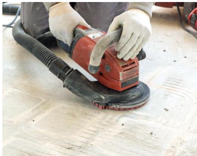
Old thinset can safely be removed when using the correct tools to control the dust created in the process.
