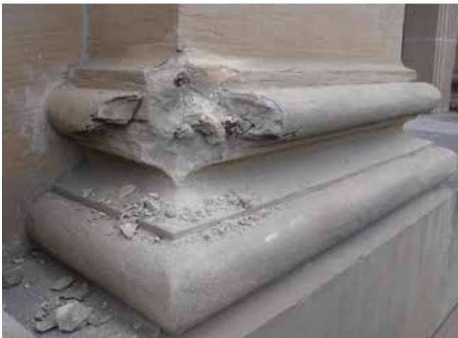
Common nails as pins and inappropriate repair mortar.
