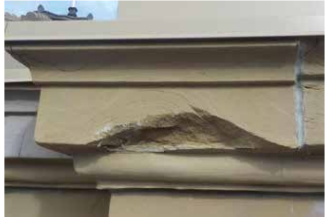
Spalled lower belt cornice stone.
