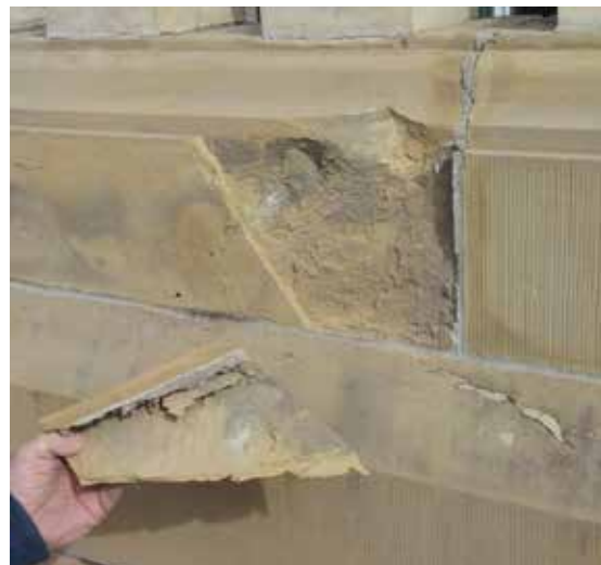
Exfoliated balustrade bottom rail.
