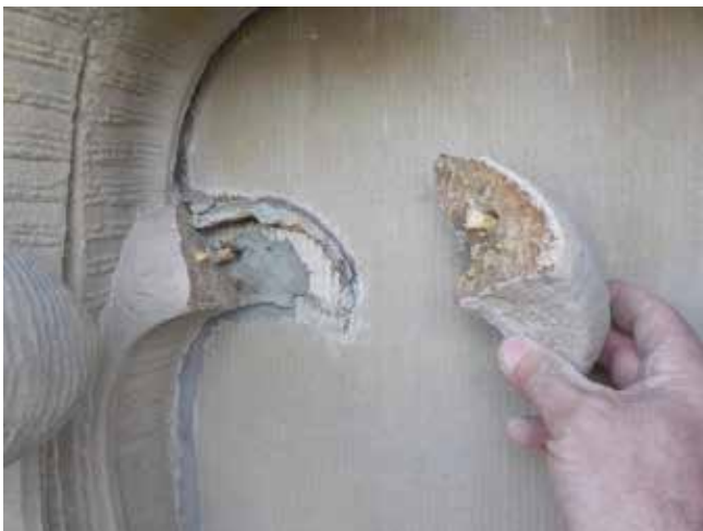
Wood dowel and inappropriate adhesive.
