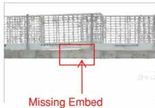
Image 2 – Missing embed located on-site.
