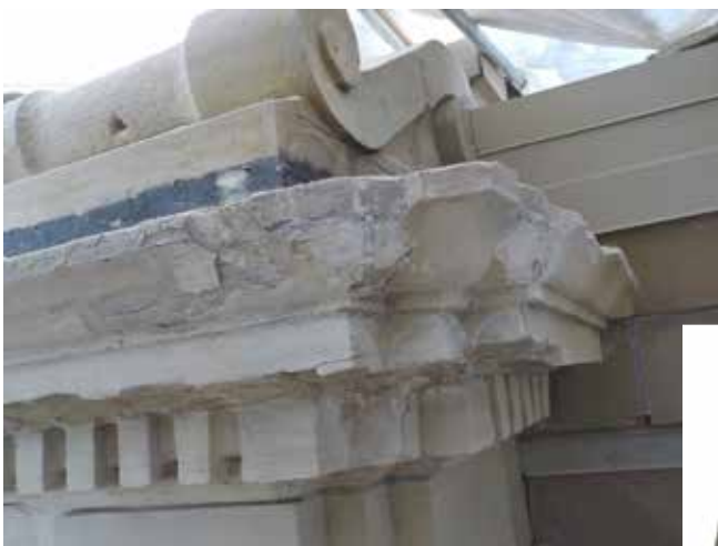
Inappropriate plastic repair of cornice stone (left) and unit replacement (right).
