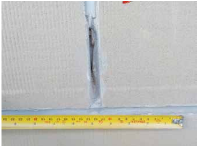
Unnecessary removal of stone arises during repointing.
