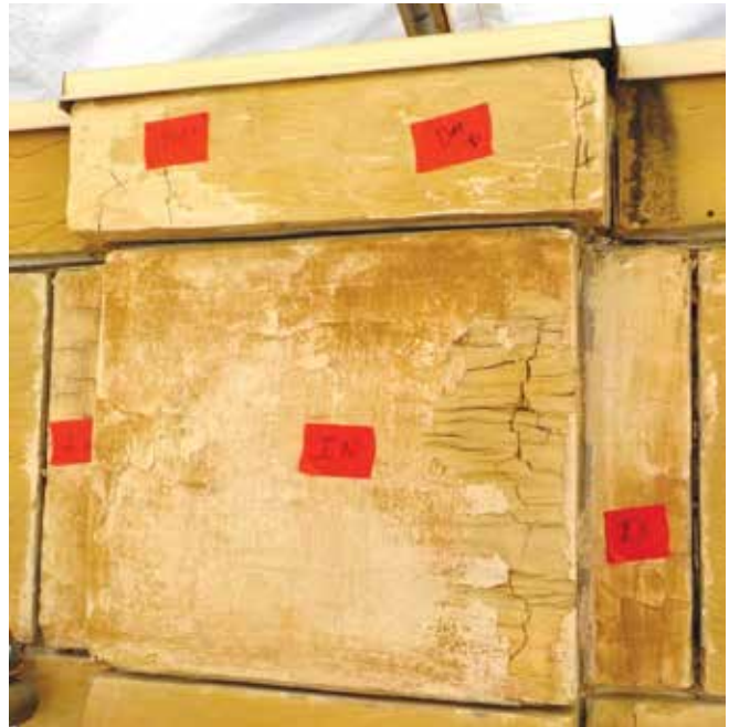
Inappropriate coating repair material and methodology.
