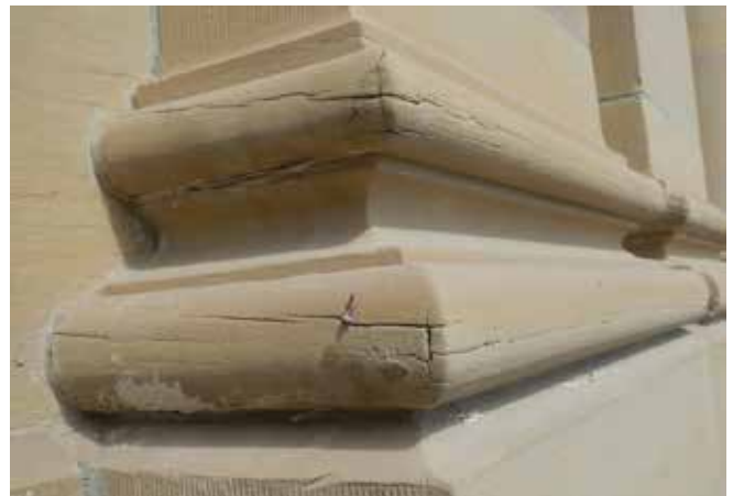
Cracked column base toruses.
