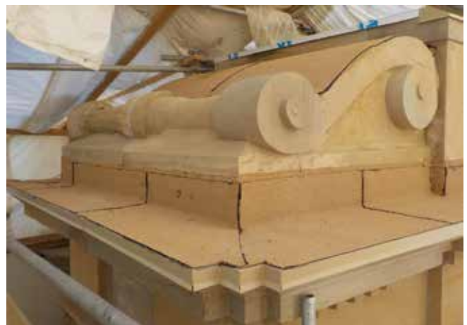
South wing roof-top scroll before and after restoration, complete with replacement membrane flashing.
