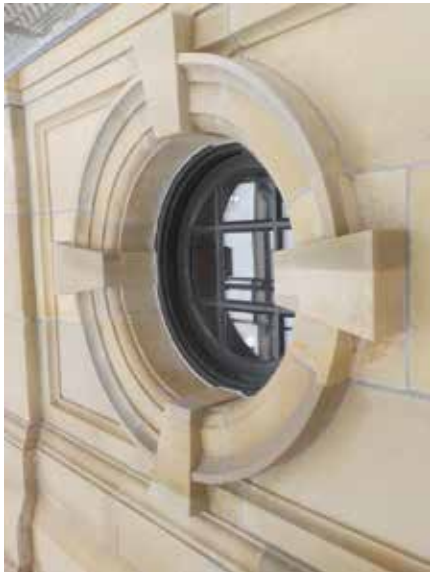
Below: South wing bull's-eye window with sandstone Dutchman interventions marked (left), repair prep work underway (middle), and interventions and window repainting completed (right).
