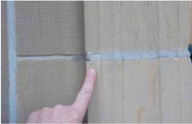
Original mortar colour and joint width (arrow) in comparison to inappropriate repointing.
