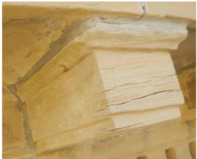
Cracked box modillion and mortared head joint.
