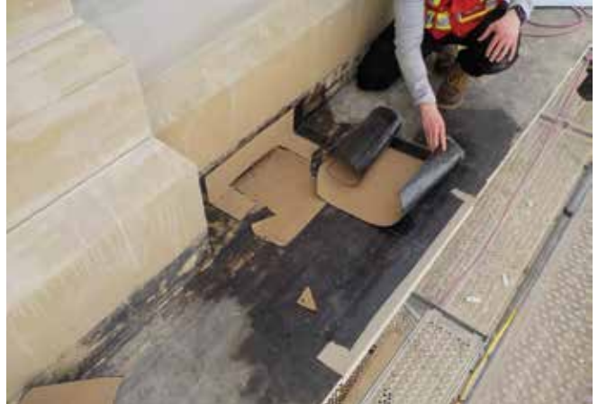
Upper cornice membrane flashing with base sheet and sheet metal nose flashing installed, ready for granulated cap sheet.
