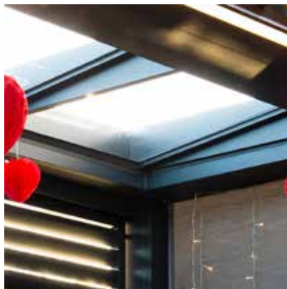
Fixed 1.5m section of glass to rear of structure provides an abundance of natural light
