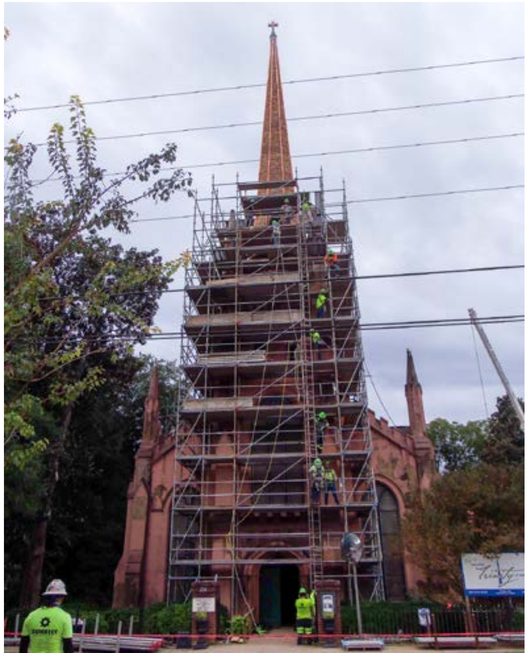
The process of restoring Trinity Church, one of Abbeville's architectural jewels, continued in 2021. The Episcopal church, which dates from the 19th century, looks down on the intersection of Church and Trinity streets. (Staff photo by Henry E. Green)
