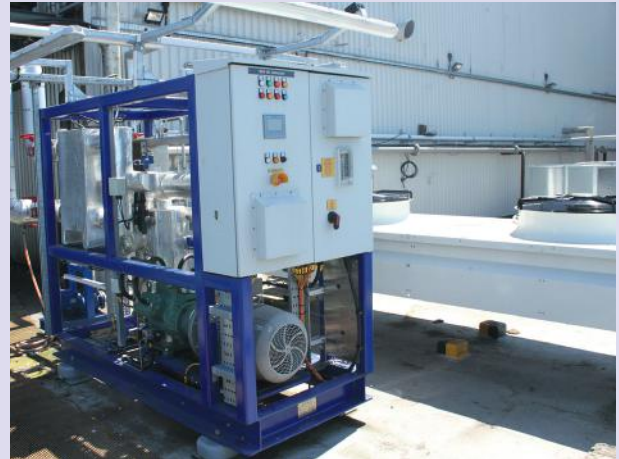
The water-cooled ultra-low charge KGM ammonia chiller at Sterling Pharma Solutions
