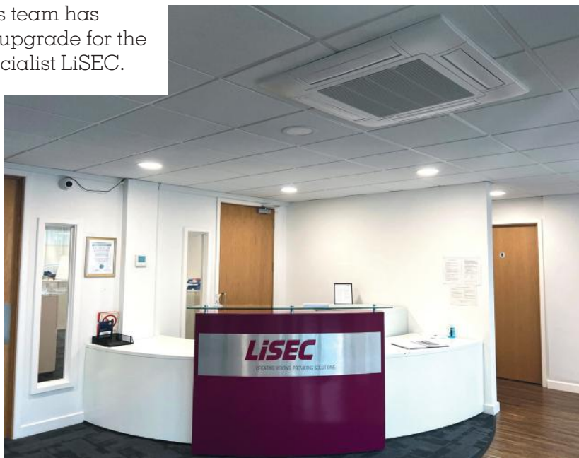
The 4-way cassettes blend in with the surrounding tiling
