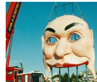
Step 5. Craning the sculpture into position and installing it on site in place of the old sculpture.
