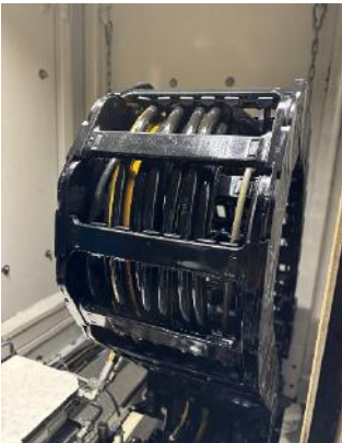
Machine Electrical parts Cleanliness
