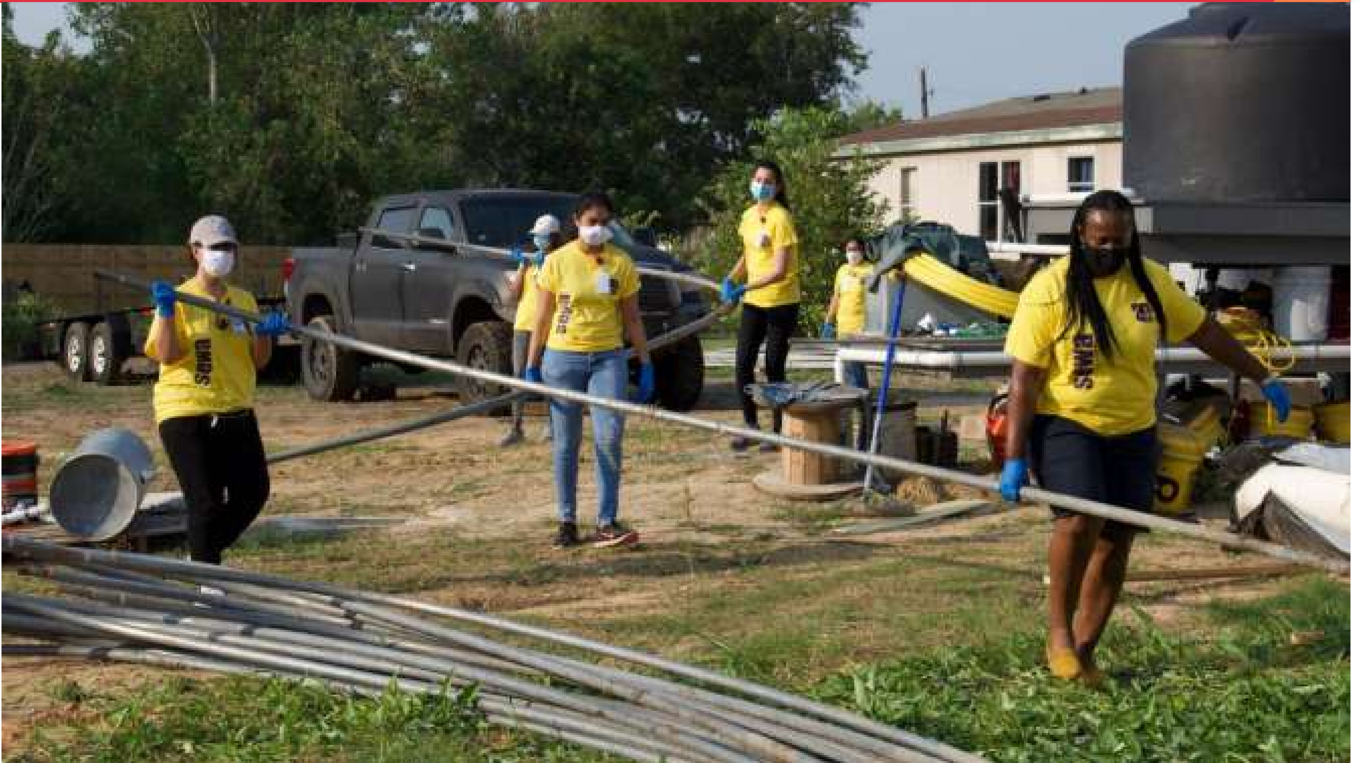
Sewa AmeriCorps Volunteers at work in Rosharon, TX. Sewa helped rebuild the Rosharon community after Hurricane Harvey hit Houston in 2017.
