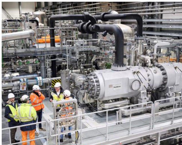
Above: A 70 MW Mega Heat Pump provides climate-friendly district heat for Esbjerg in Denmark. © DIN Forsyning/Christer Holte.
