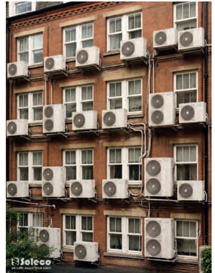
Increasing installation density raises the risk of structure-borne noise
